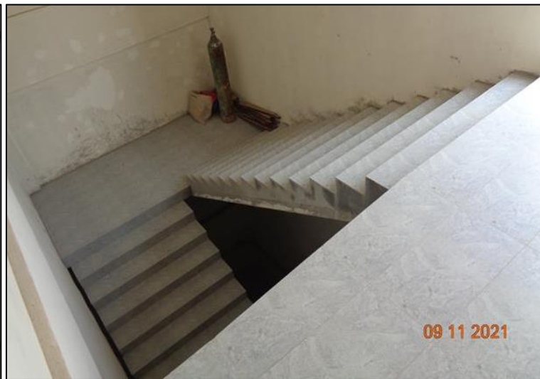
Missing railing at stair
