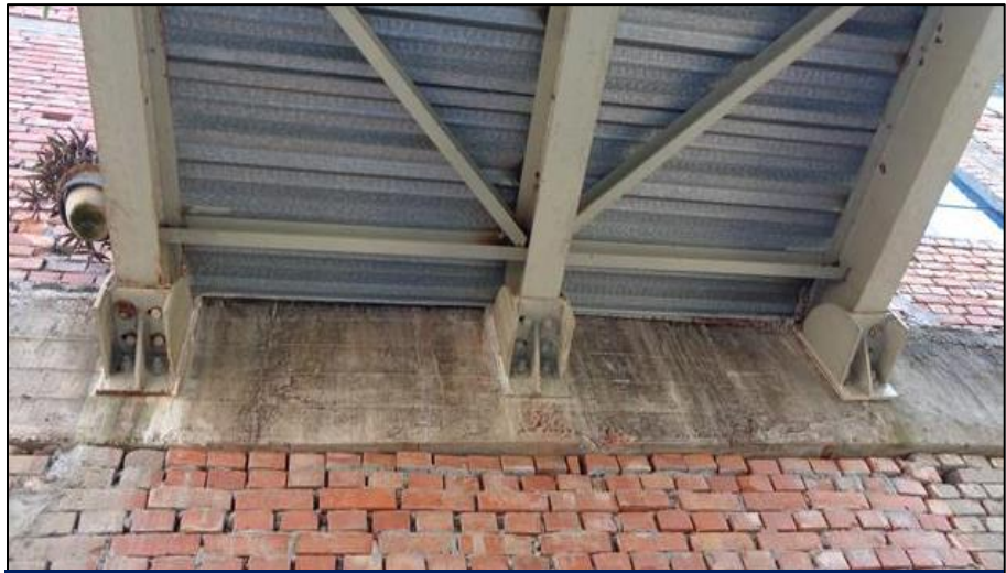
The connecting bridge was found connected with RC beam of the Famkam printing building.
