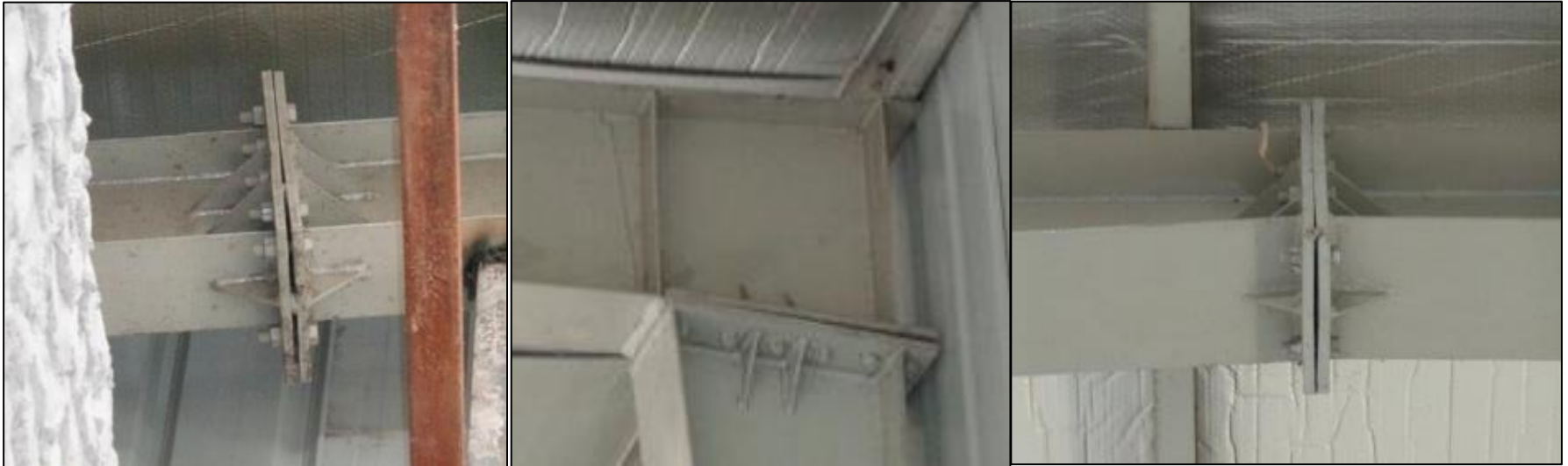
Connection gap was found in rafter-rafter & rafter-column connection
