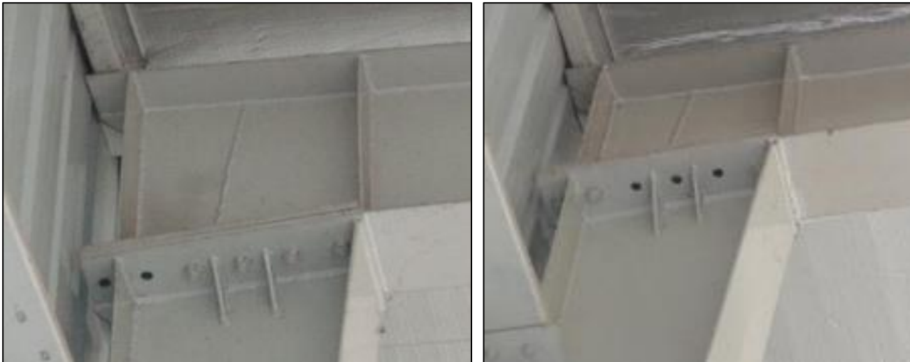
Bolt missing in Beam-column connection at ground floor
