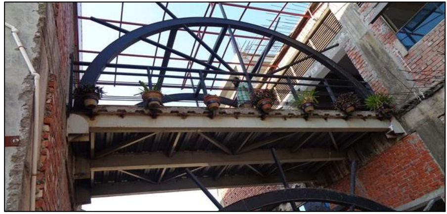
Undocumented steel connecting bridge was found. Building engineer is required to update the as-built drawing with the accurate on-site condition.
