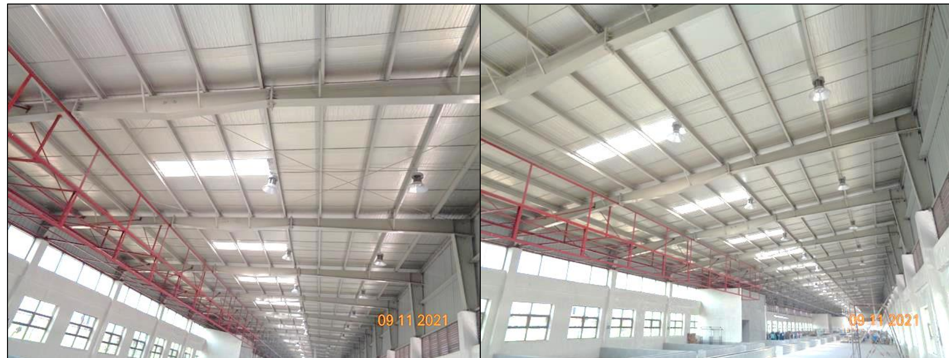
Portal steel roof shed - Lateral load transfer media missing at roof level
