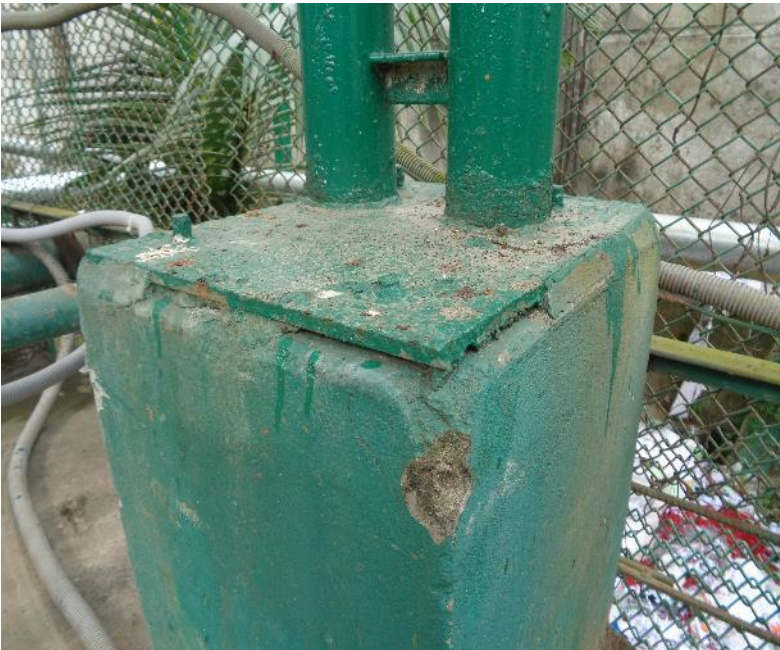
Poor connection with pedestal column
