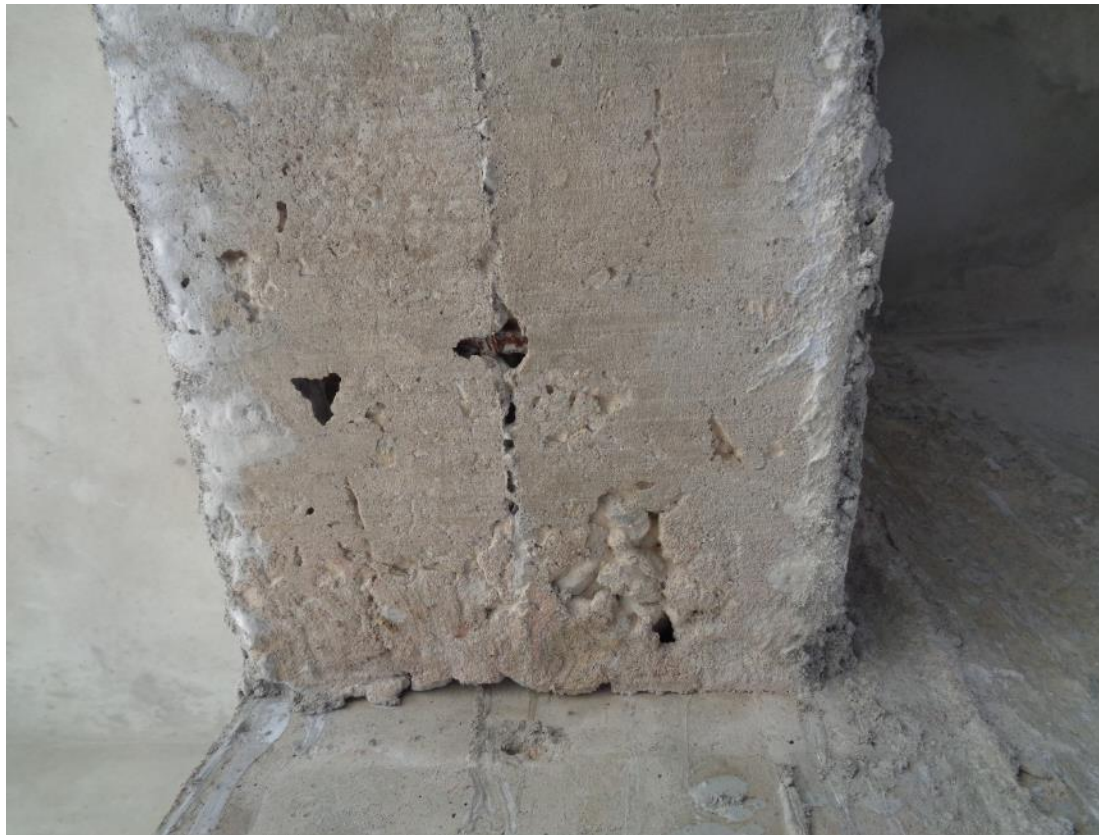
Honeycomb observed in stair roof beam
