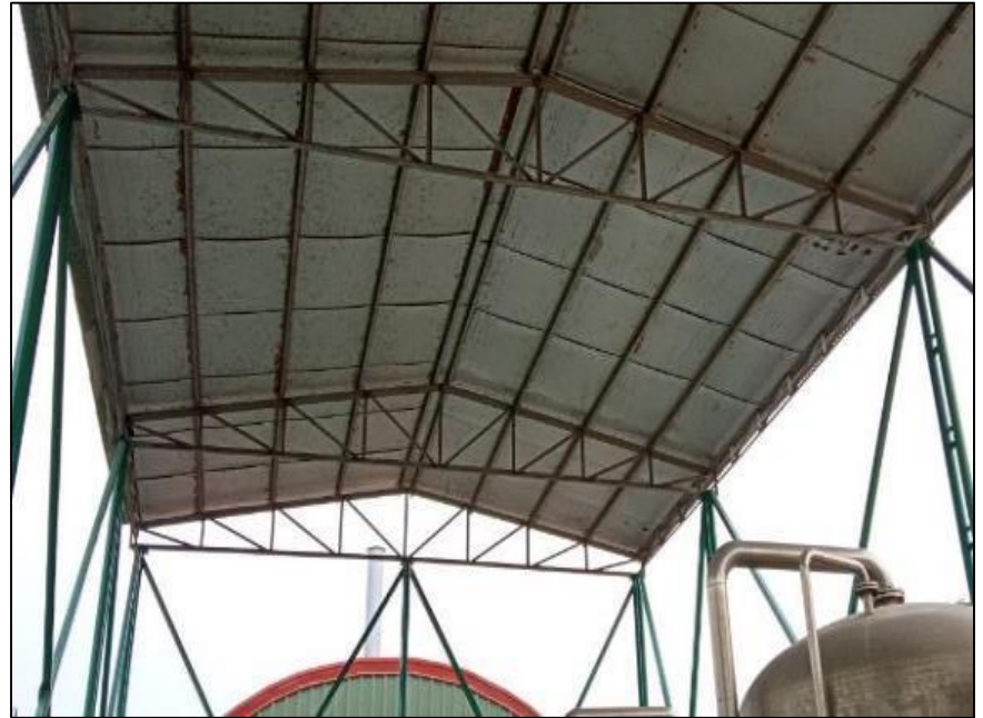
No roof bracing provided
