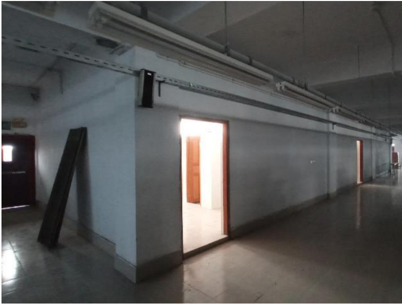
Undocumented toilet block on typical floor
