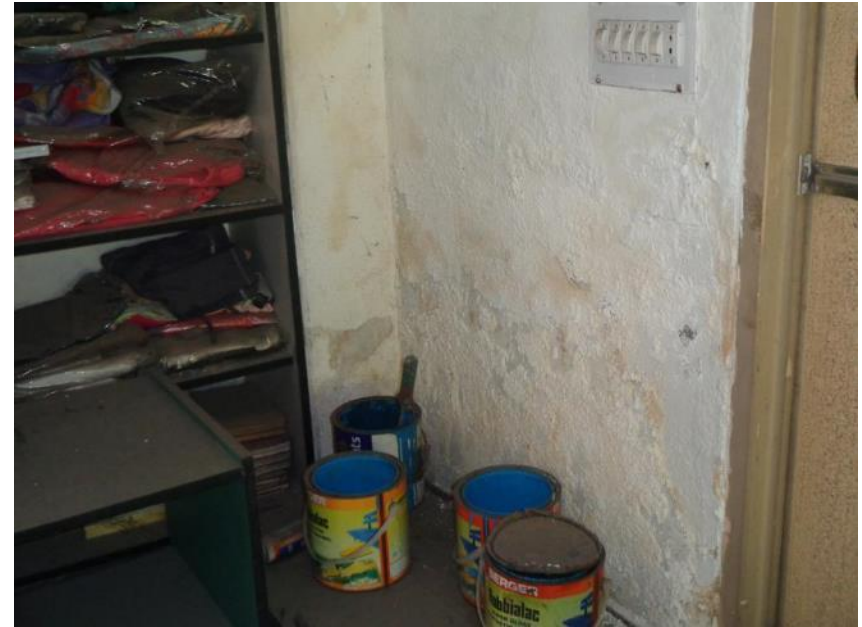
Signage of dampness at partition wall at toilet
