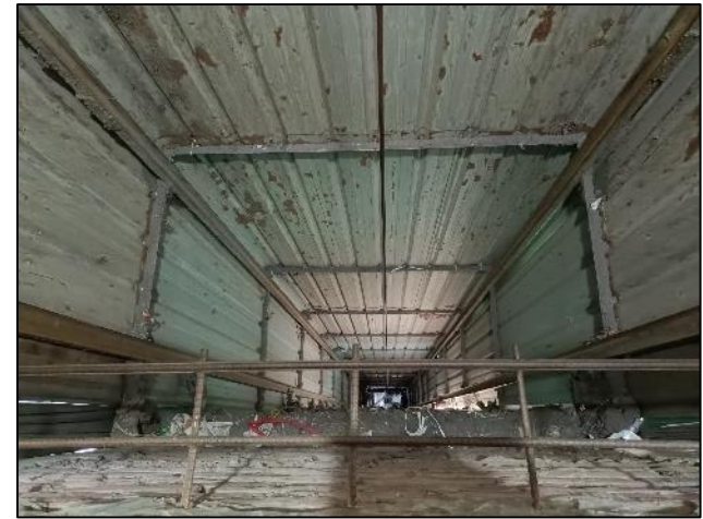
No bracing observed from inside the lift
