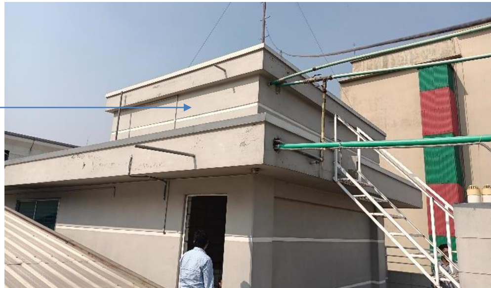
Over Head Water Tank
