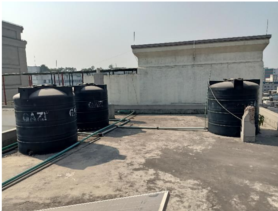
Plastic water tank on roof
