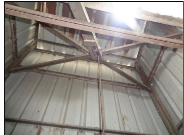
Pulley hoist of the lift
