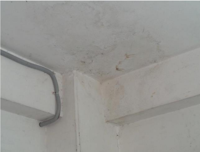
Signage of dampness at slab, beam & column
