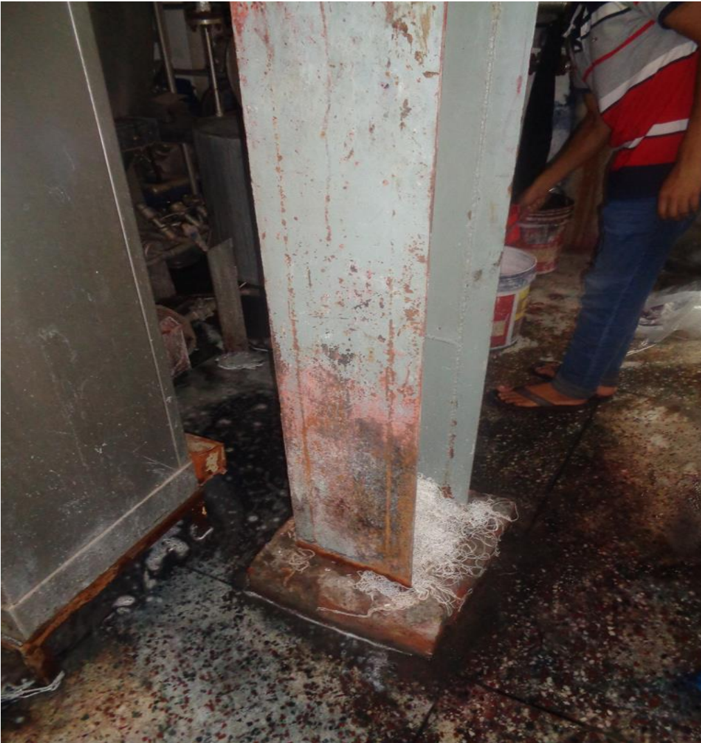
Corrosion on steel member
