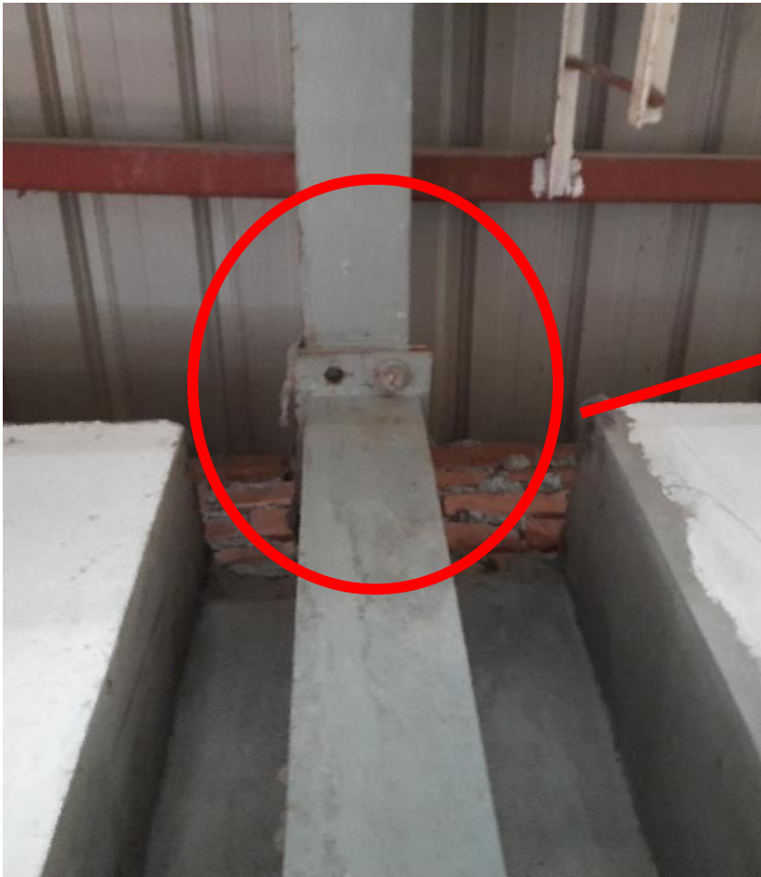
Missing bolt in steel column and rafter joint
