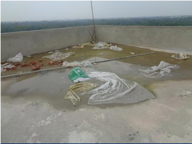
Standing water on roof
