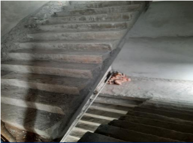
Stair without handrail
