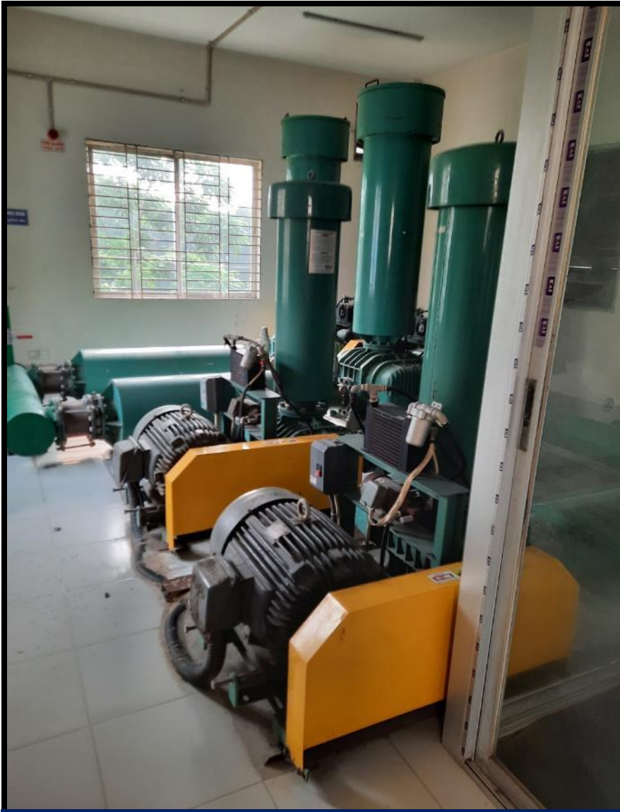
Air blower machine at 1 st floor of ETP building
