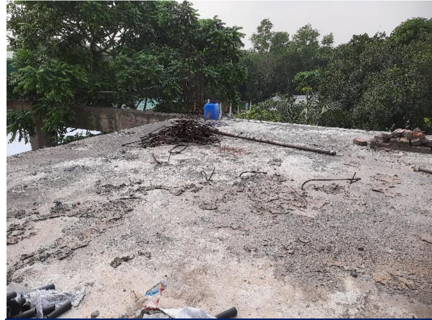
Missing parapet wall
