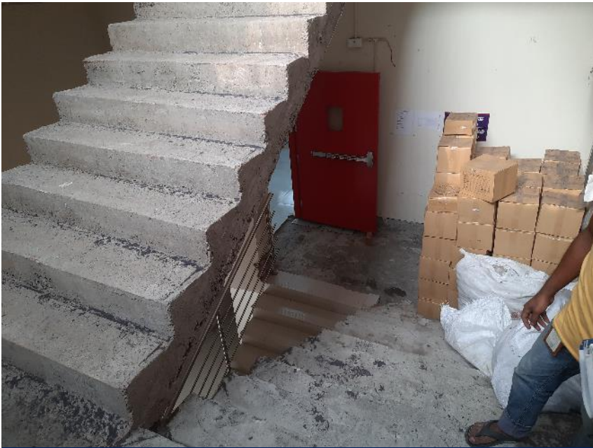
Missing stair railing
