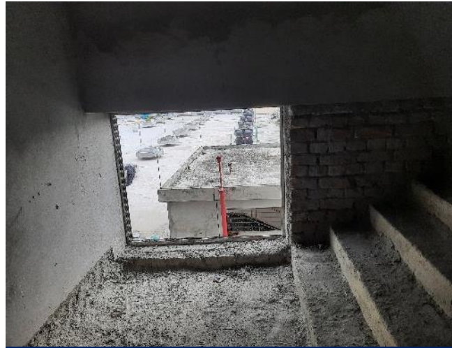
No window grill installed at stair
