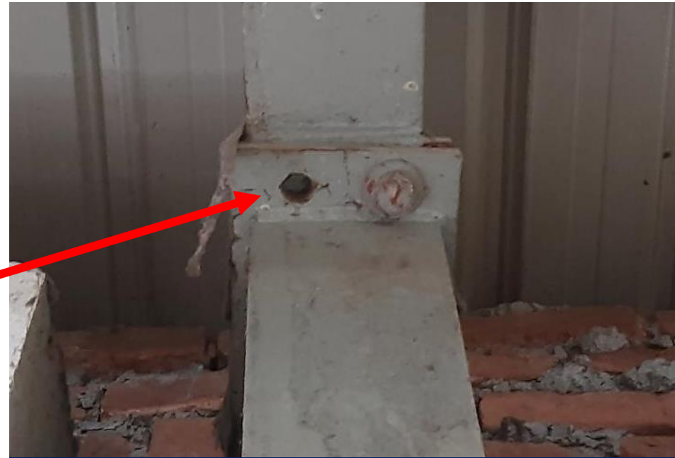
Building is required to install the missing bolt of the steel structure.
