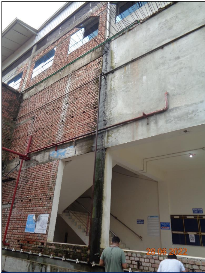
Dampness in RC Column
