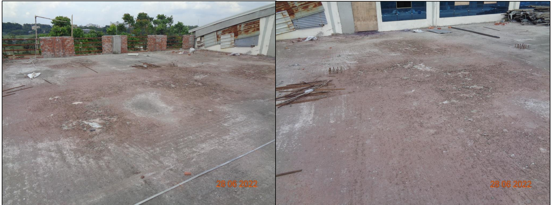
Lack of water proofing on roof slab
