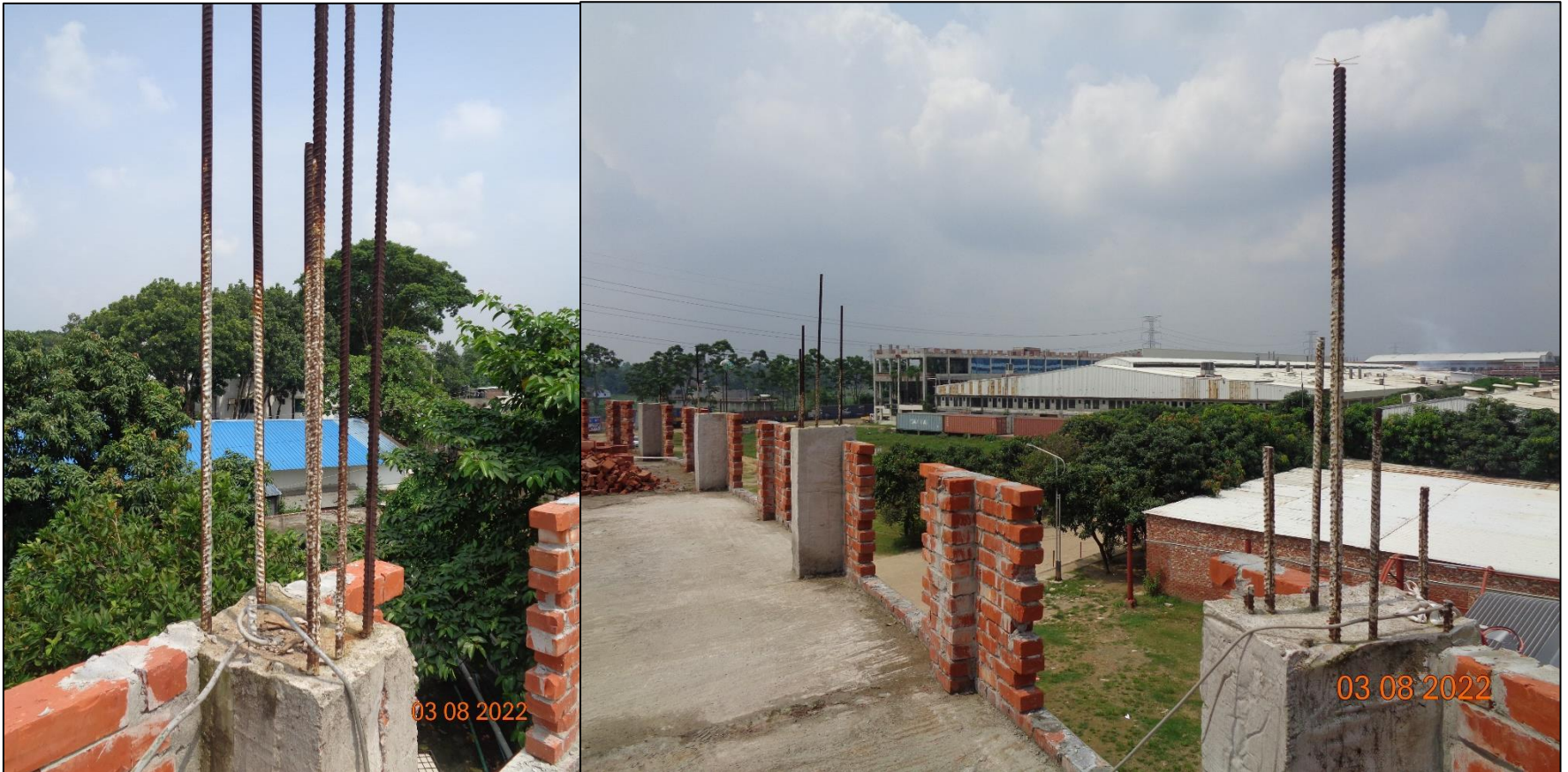
Exposed rebar at roof
