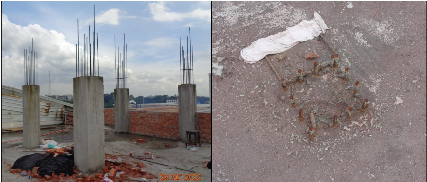
Exposed rebar at roof
