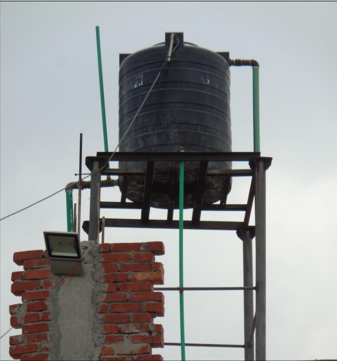
Plastic water tank at roof
