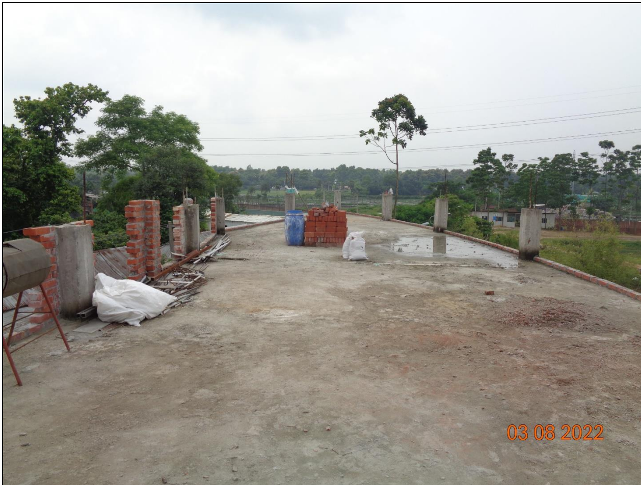
Parapet wall missing at roof
