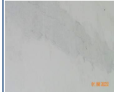
Dampness was observed in several places on the 1 st floor.
