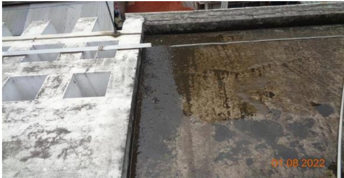
Water clogging on roof
