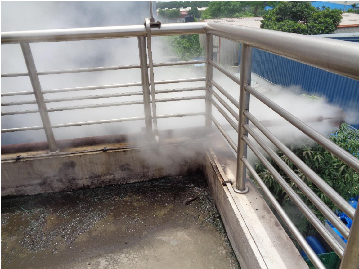
Steam flow adjacent to periphery beam
