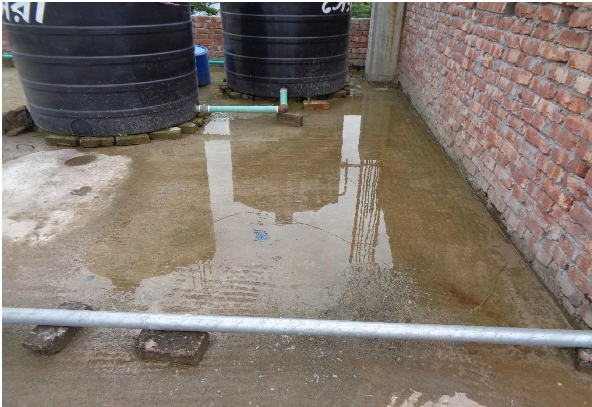
Water ponding on roof slab
