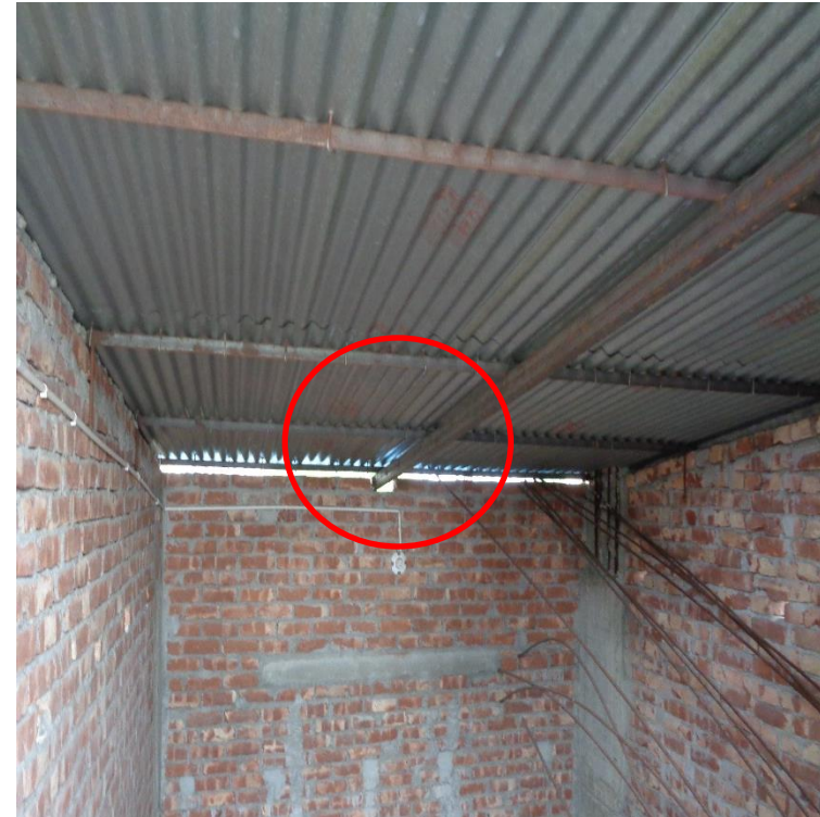
Apparently inadequate connection
