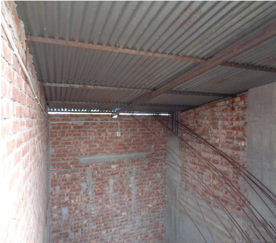
Exposed reinforcement left at Staircase
