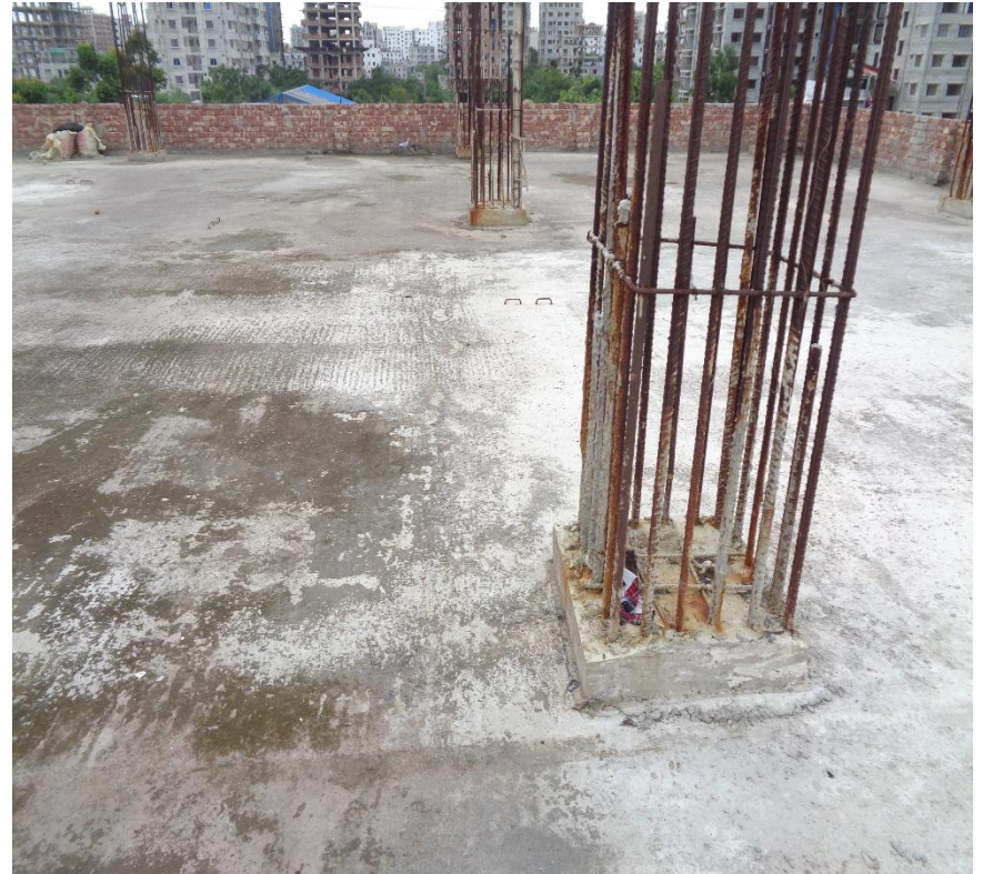
Exposed reinforcement left at roof
