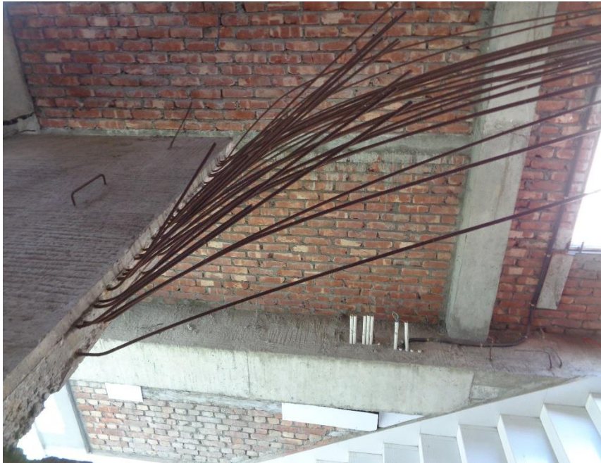
Exposed reinforcement left at Staircase
