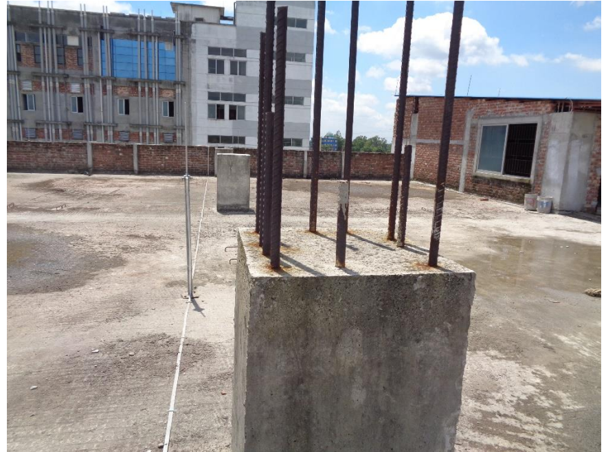
Exposed reinforcement left in column at roof
