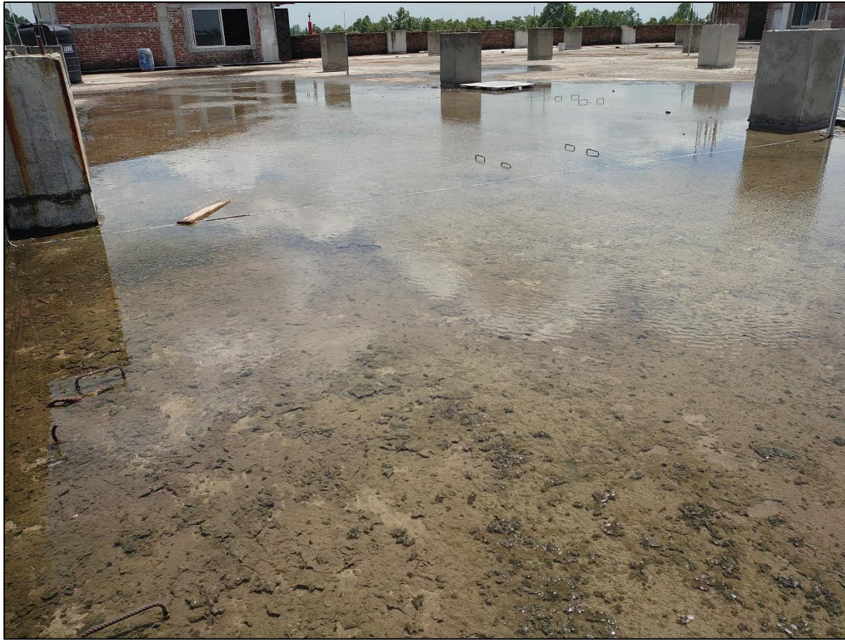
Water ponding on the roof slab
