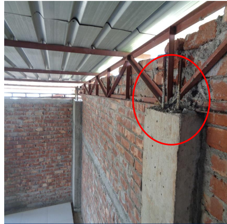
Roof truss not anchored with the rebar of RC column
