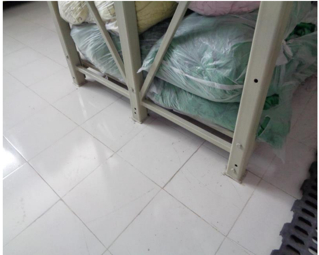
Rack without lateral bracing or anchorage
