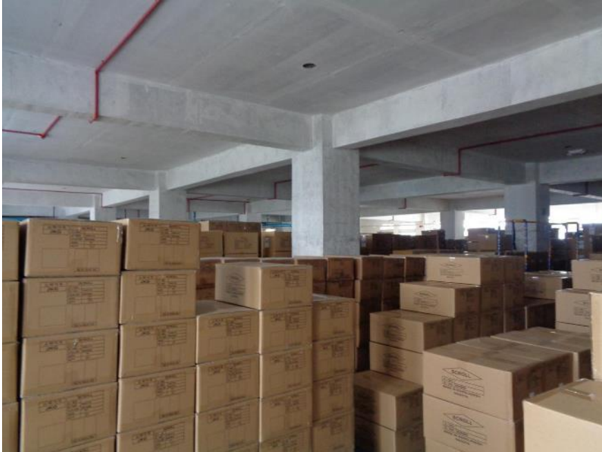
No load height marking on 2 nd floor storage area
