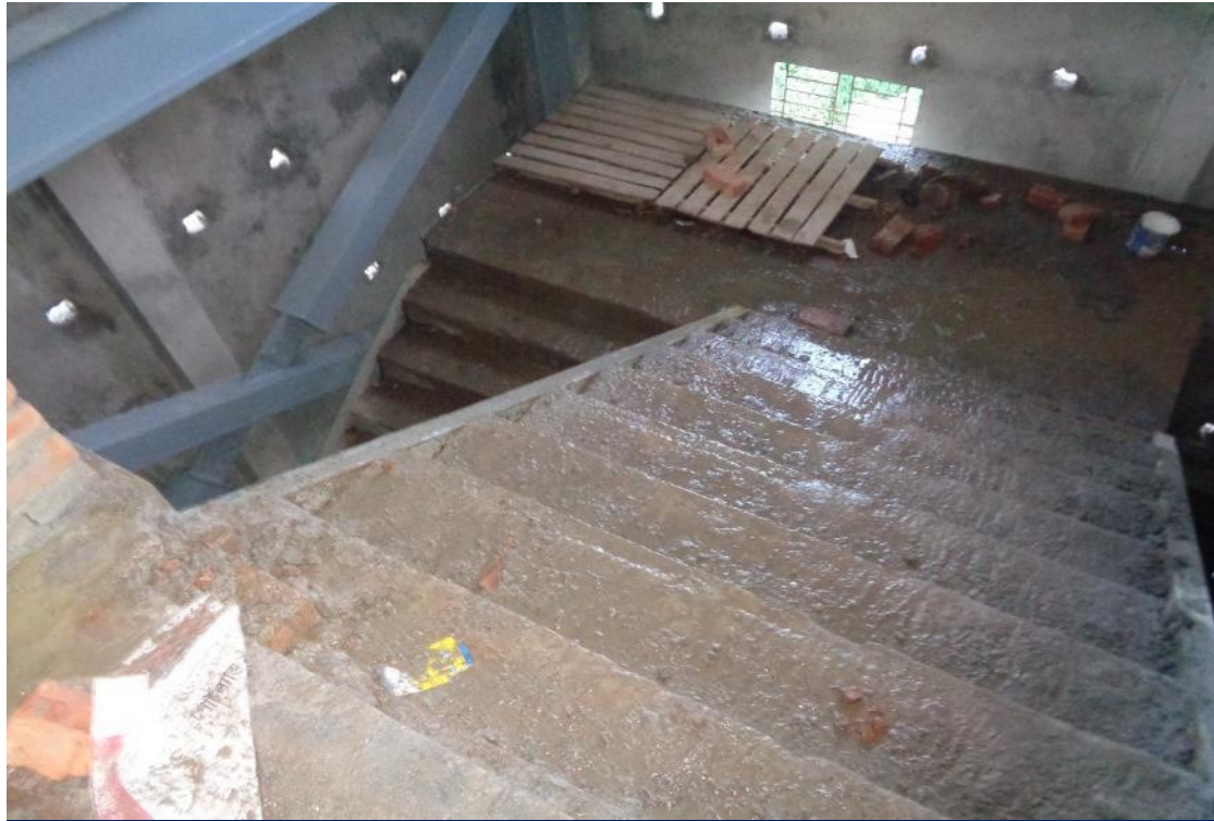
Railing was missing at several location at staircase
