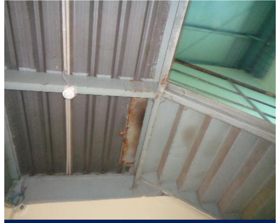
Corrosion on steel members
