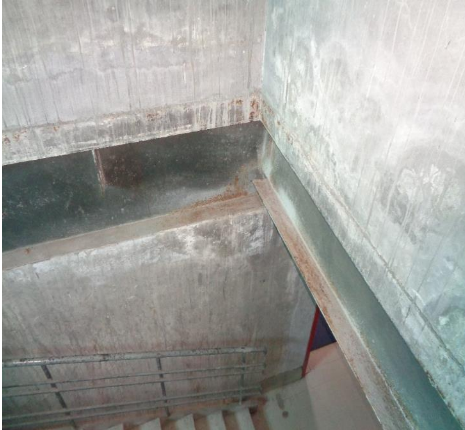
Corrosion on steel members
