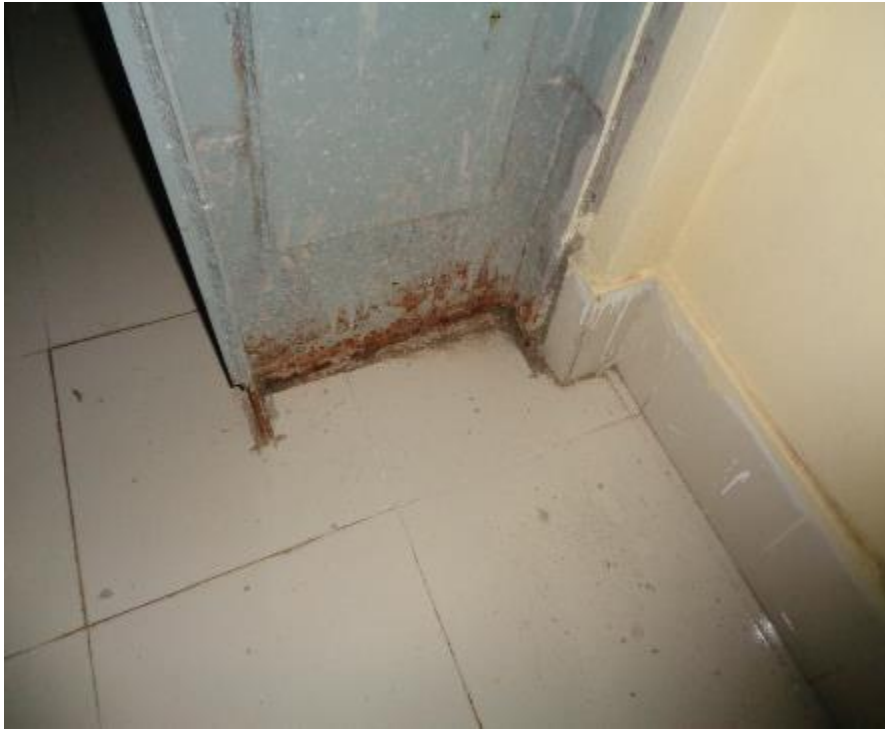
Corrosion on steel members
