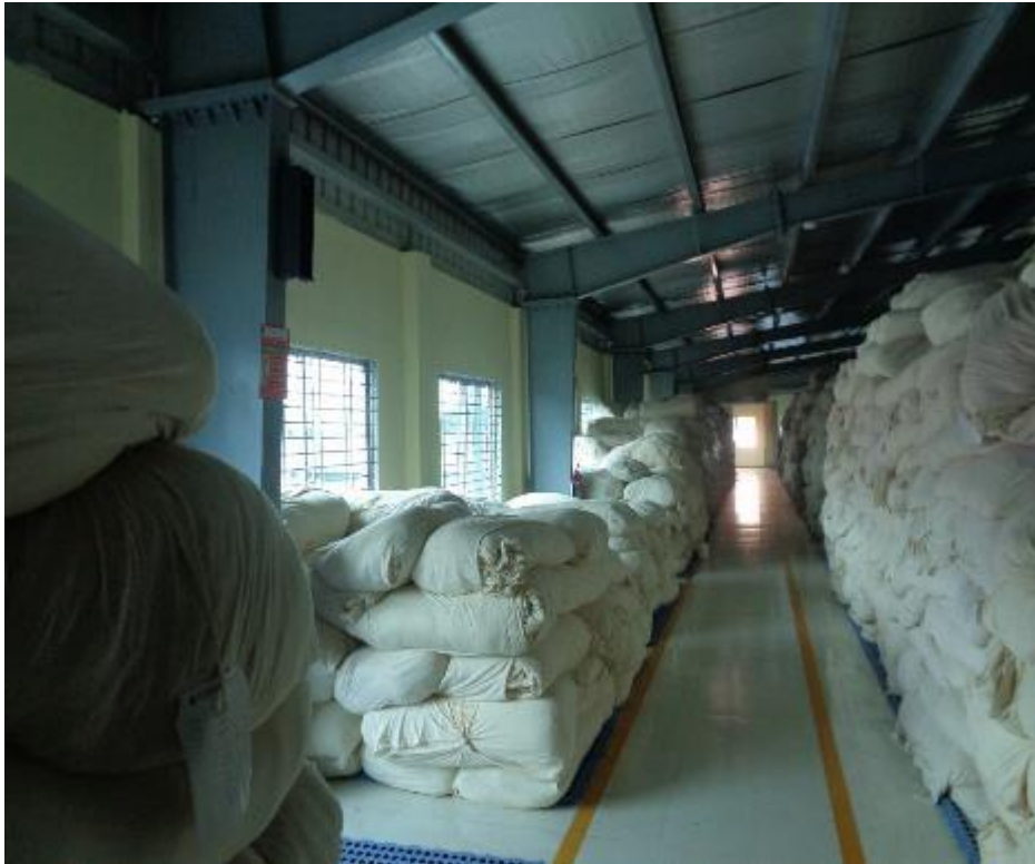
Load transfer media is missing at most of the location along long direction
