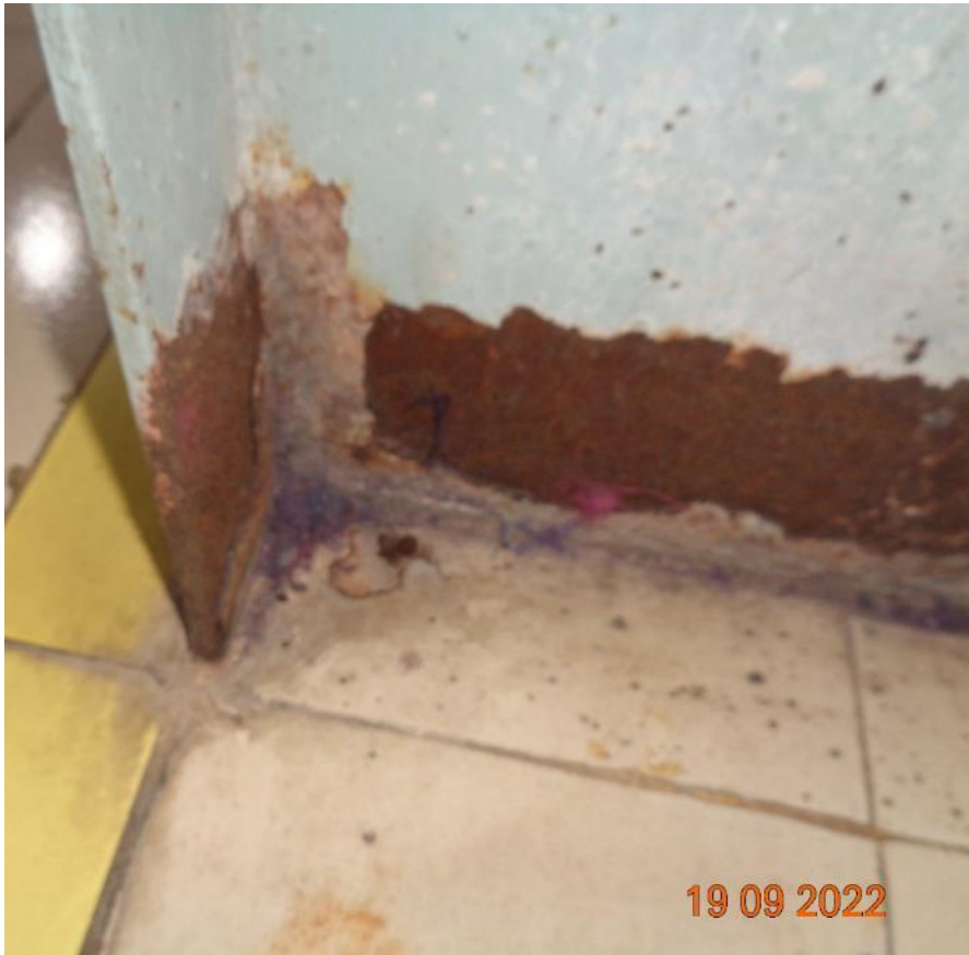
Corrosion on steel members
