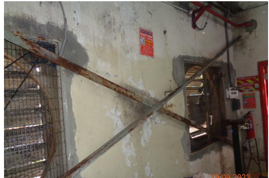
Corrosion on steel members
