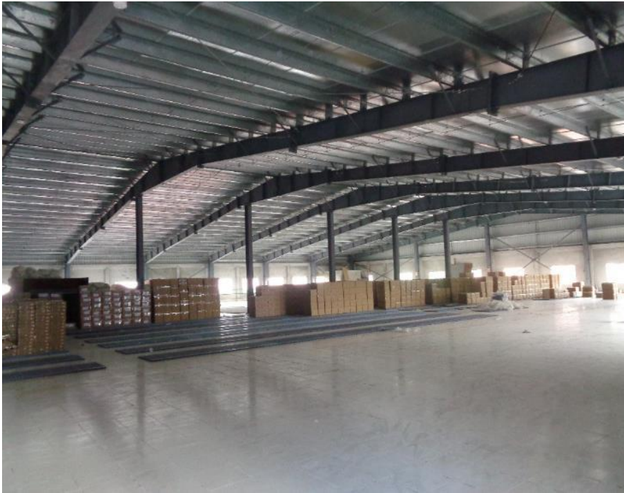
One internal column found at every grid along ridge at first floor
