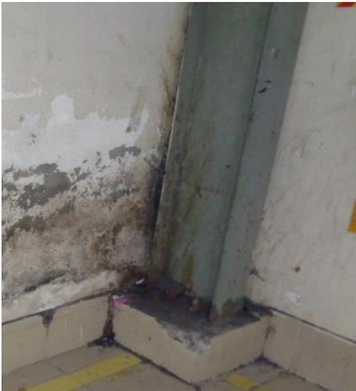
Retrofitting work is not implemented
