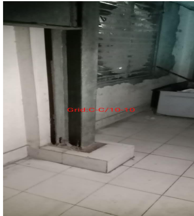
Retrofitting work is not implemented
