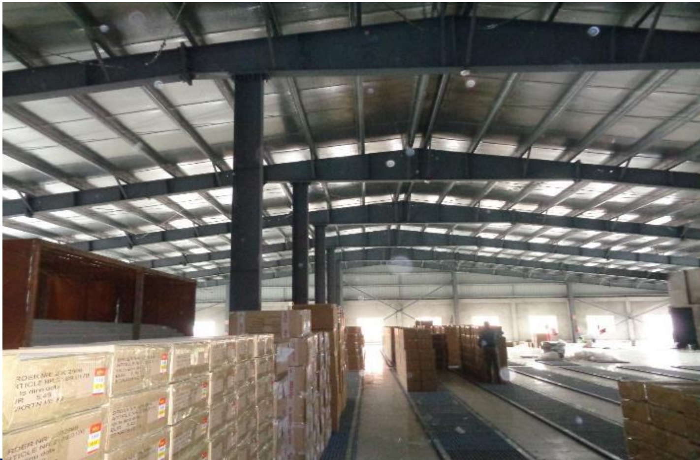
Column not placed along ridge
