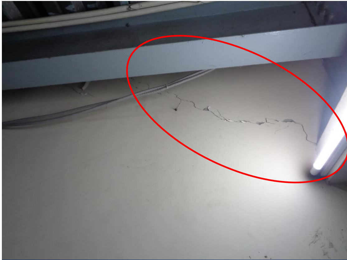
Crack observed on brick wall at several locations
