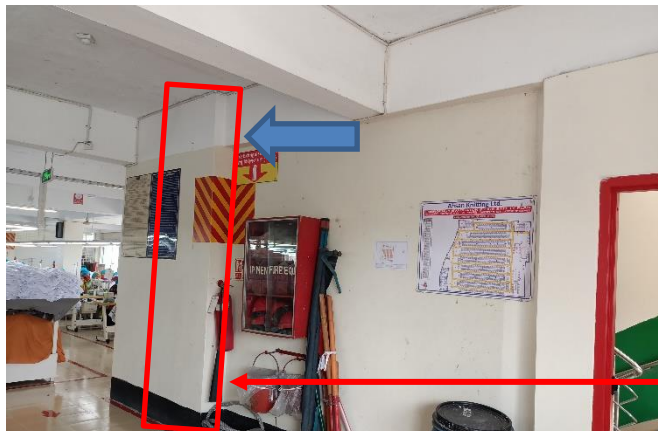
Column found offset from beam-column joint
