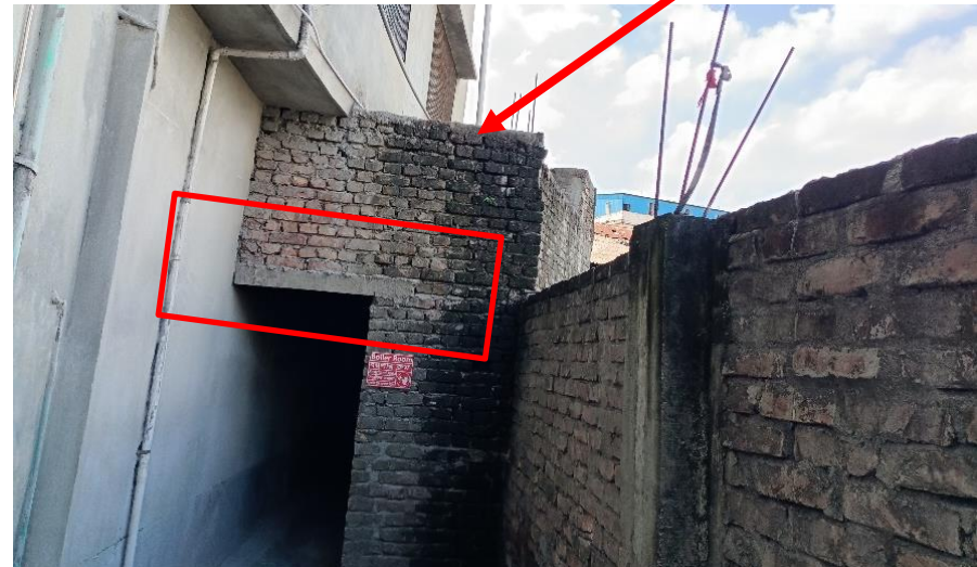
Unsupported Lintel in Boiler & Generator Room
