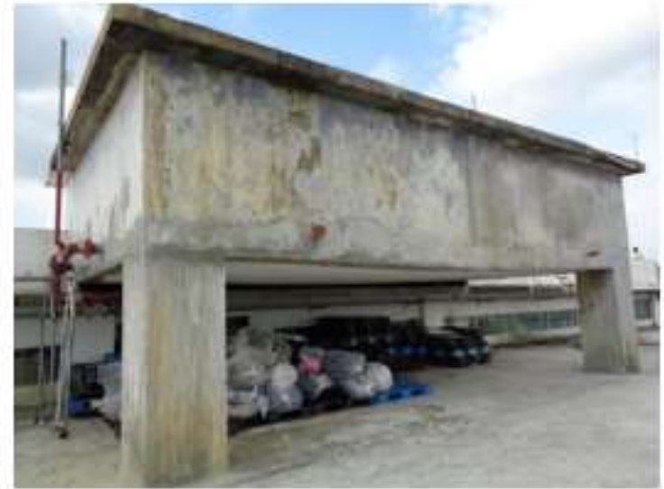
Deflection at slab
