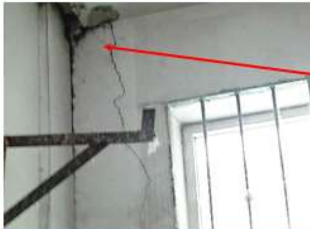
Zoom view of crack
