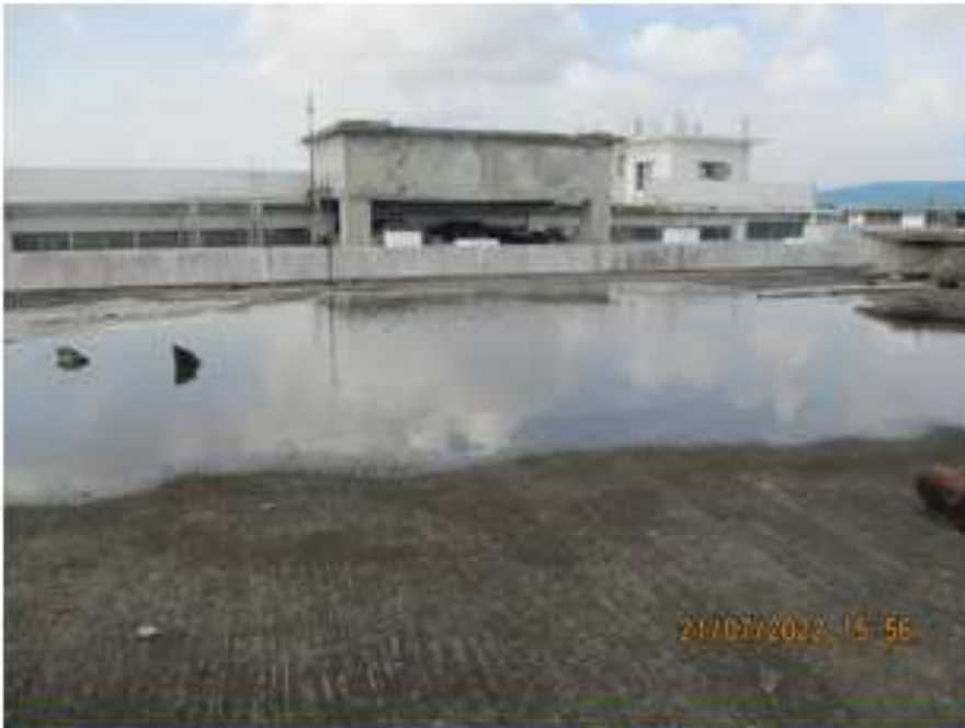
Standing water on the roof of RO plant
