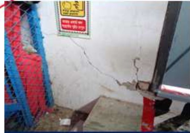
Cracks on wall
