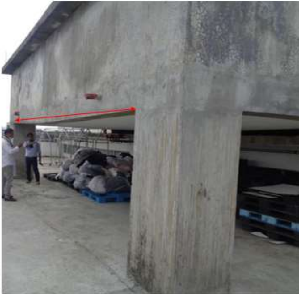
Deflection at Inverted beam of OHWT
