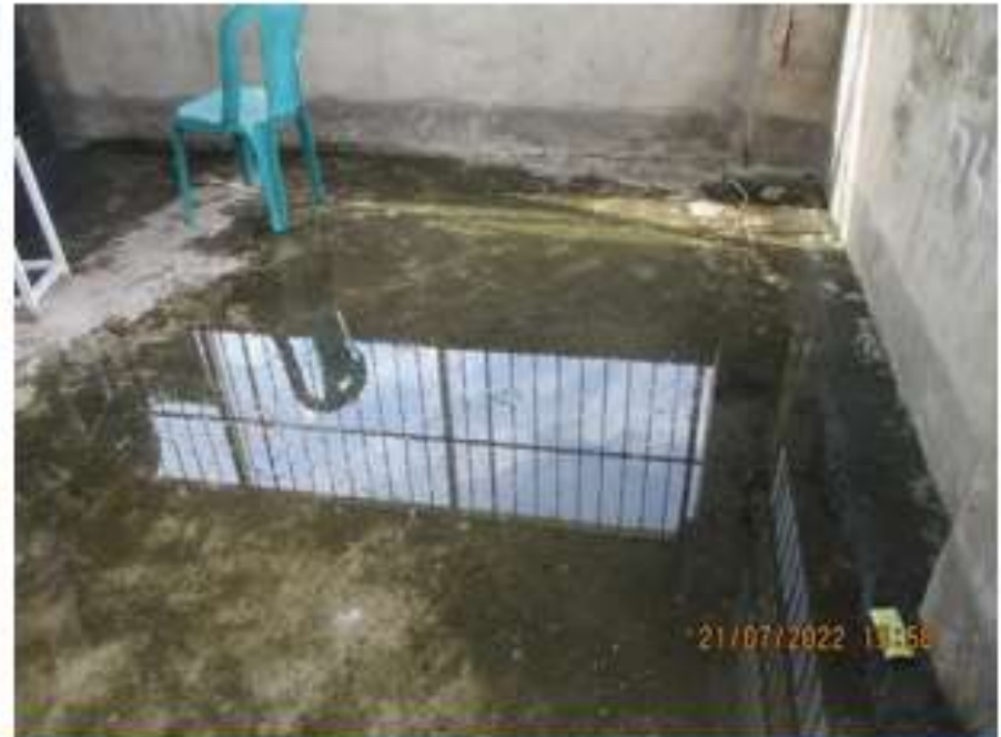
Standing water on the floor of RO plant
