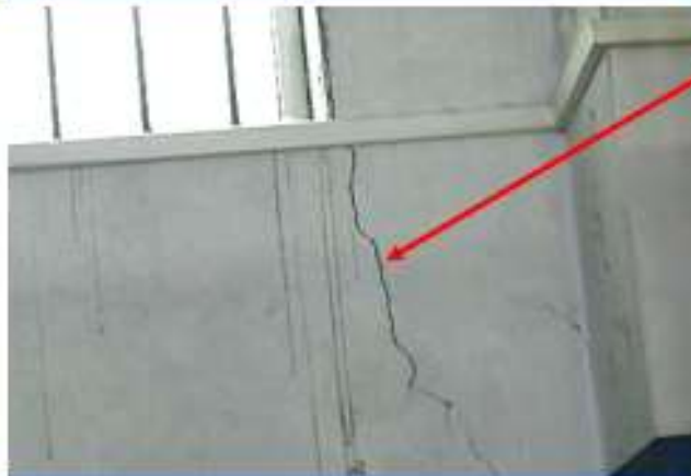
Zoom view of crack
