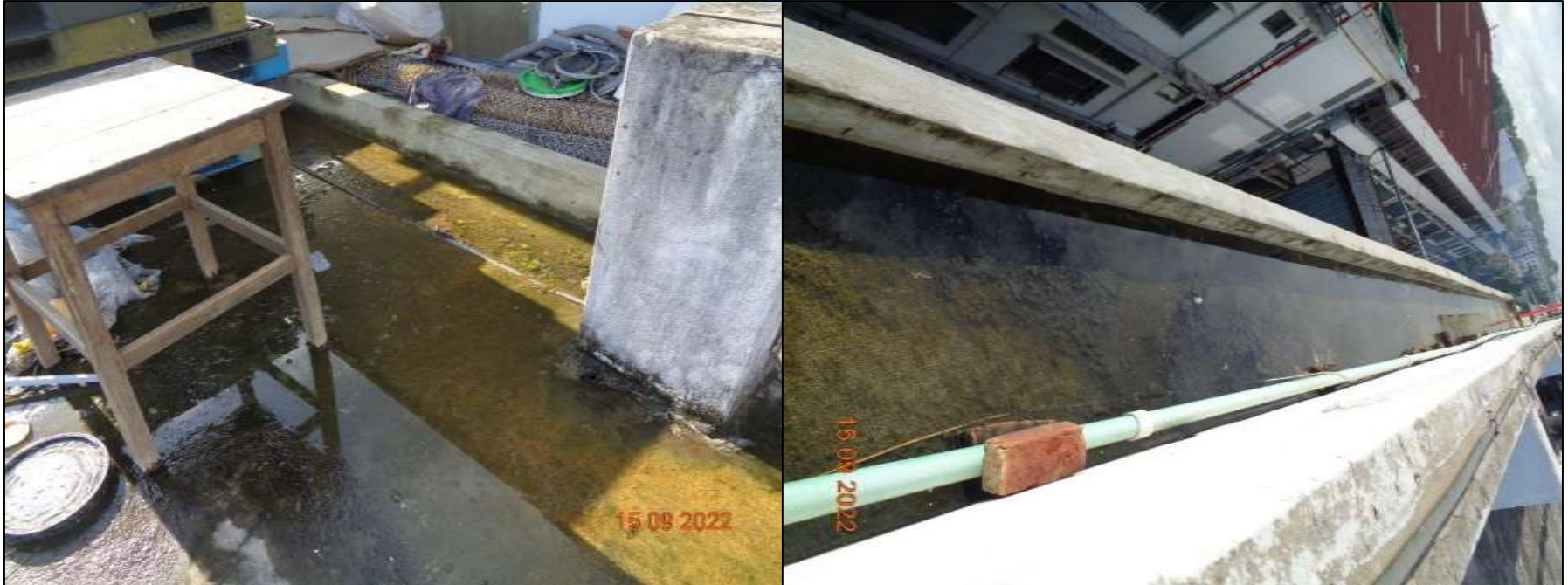
Water ponding at Roof
