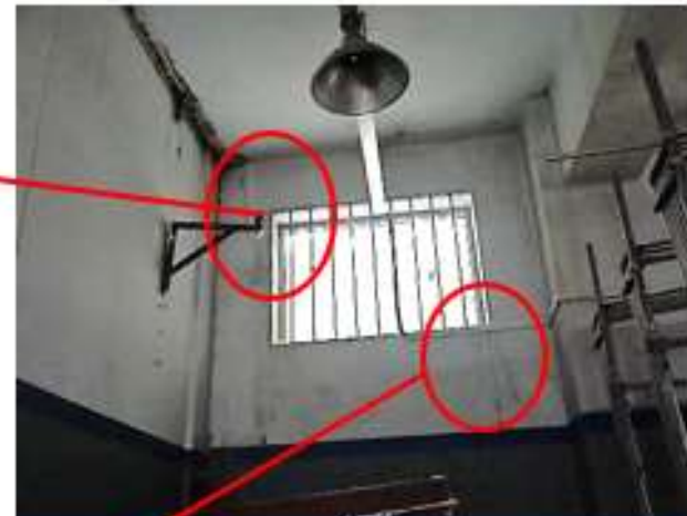
Cracks on wall
