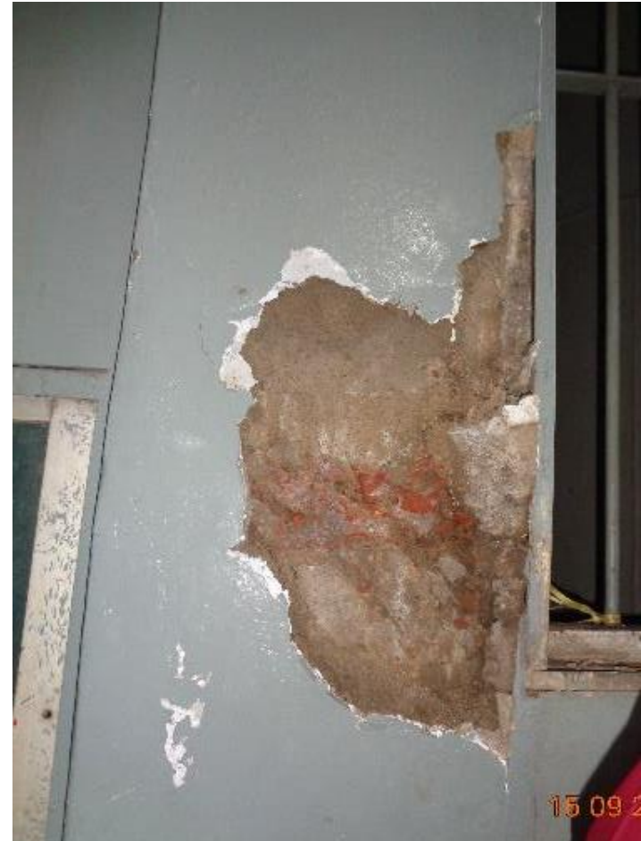
Brick chips at column (Block-B)
