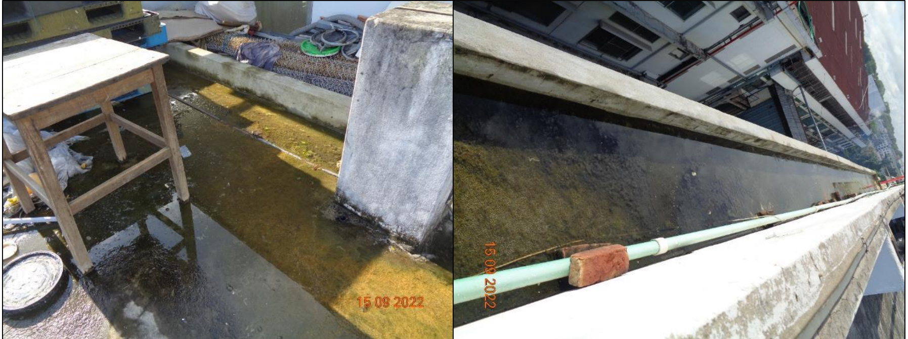
Water ponding at Roof
