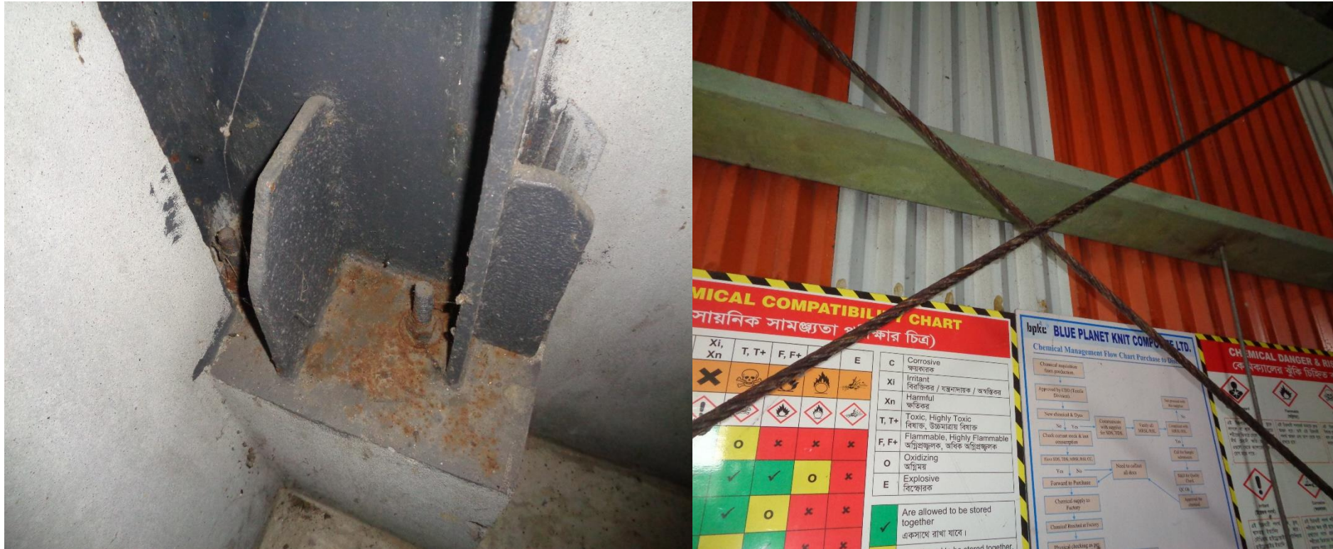
Corrosion on steel member and cable bracing
