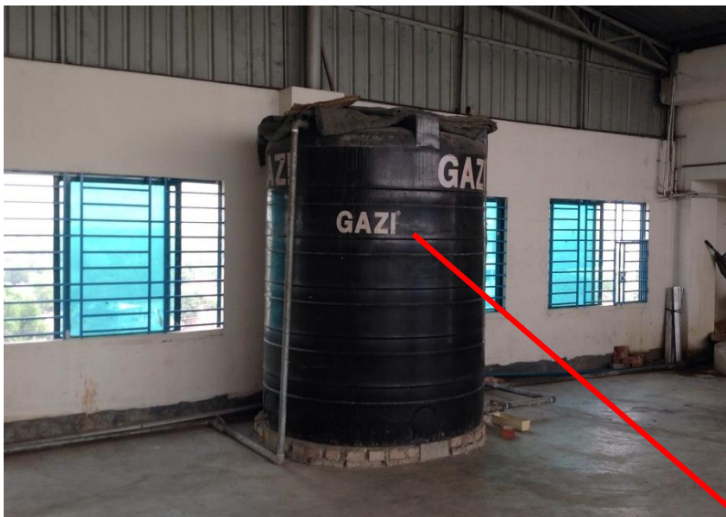
Roof – Plastic Water Tank
