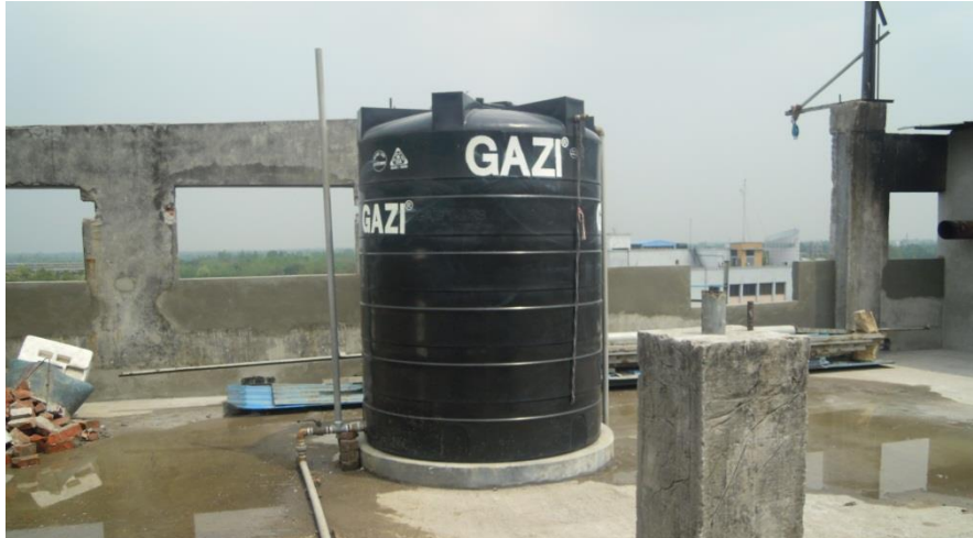
Ponding to Roof
