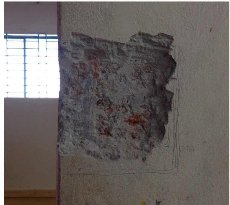
Tested Ground Floor Column C2 (2007) Brick Aggregate Noted.
