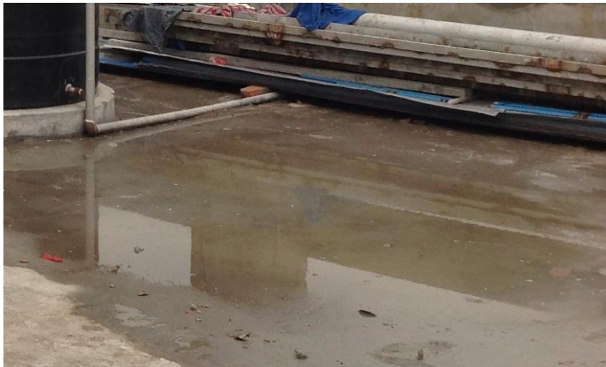
Ponding to Roof
