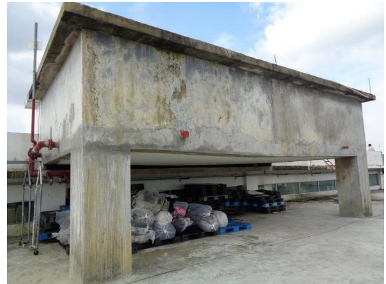
Deflection at slab
