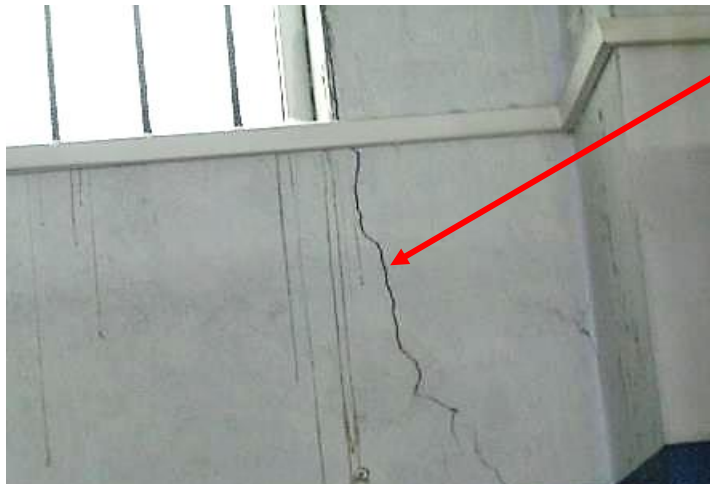
Zoom view of crack
