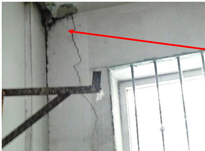
Zoom view of crack
