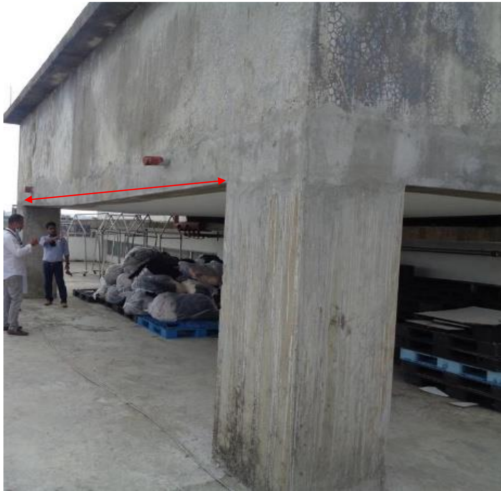
Deflection at Inverted beam of OHWT
