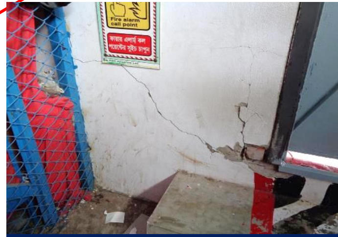
Cracks on wall
