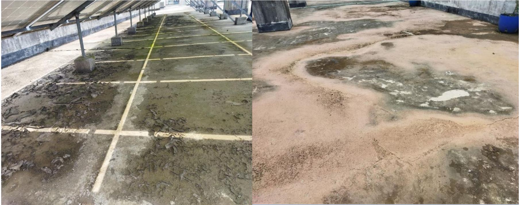
Signage of water ponding on roof slab
