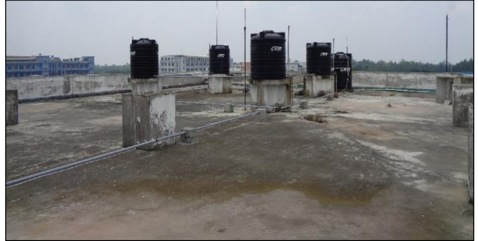
Signage of water ponding
