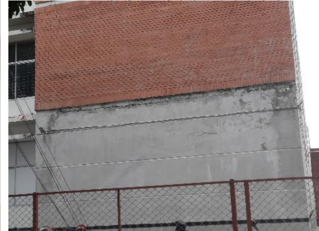
Crack in the façade wall
