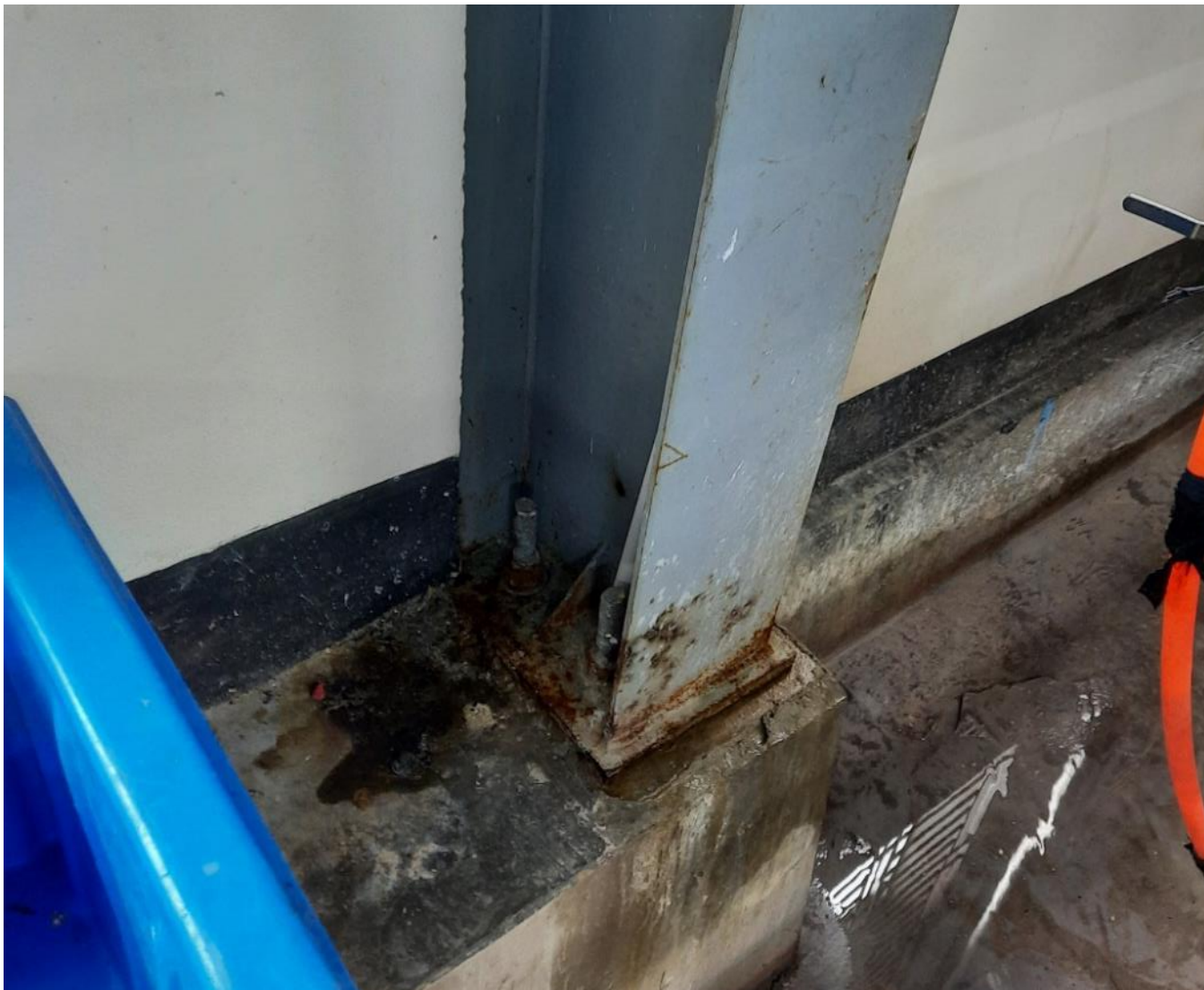
Corrosion in steel column
