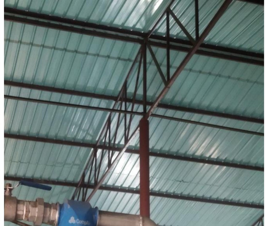
Poor connection at truss to column
