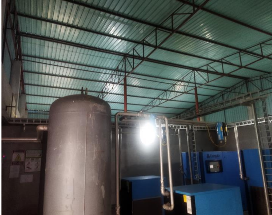
No bracing system/load transfer media provided
