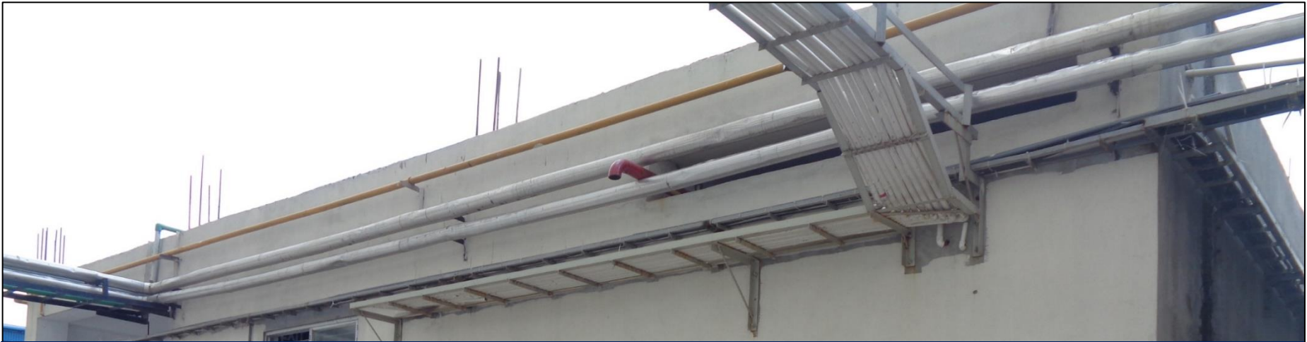
Exposed rebar of column
