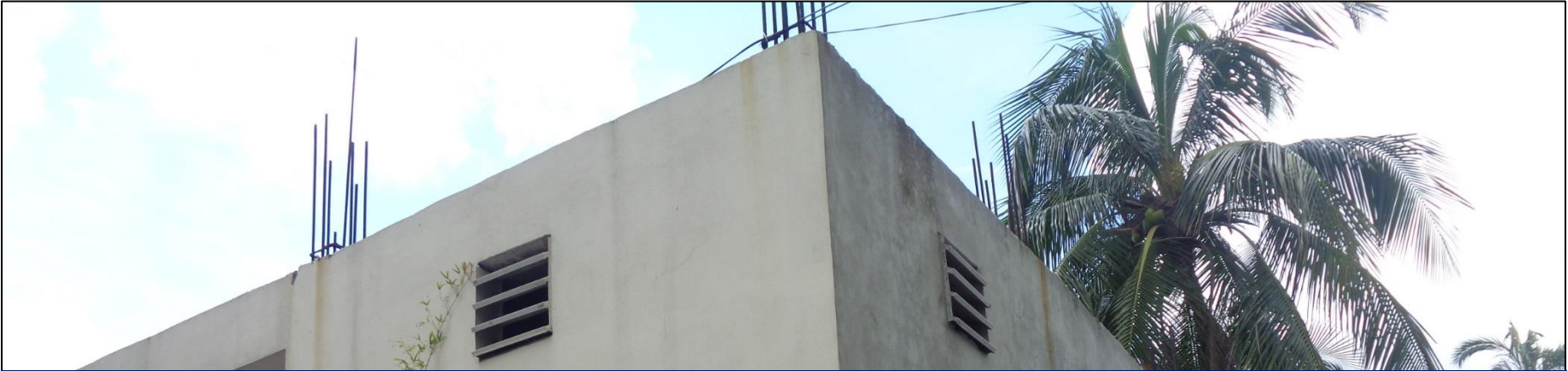
Exposed rebar of Column
