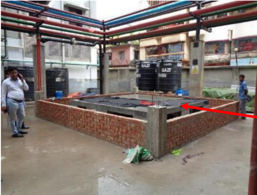
Undocumented rooftop slab and column on site
