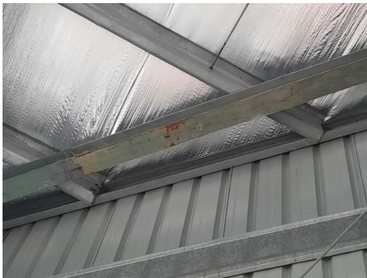
Corrosion on steel column
