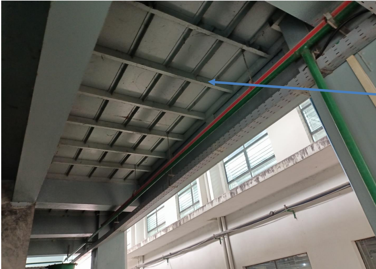
Undocumented Deck slab
