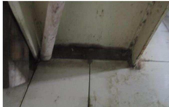
Corrosion on steel column
