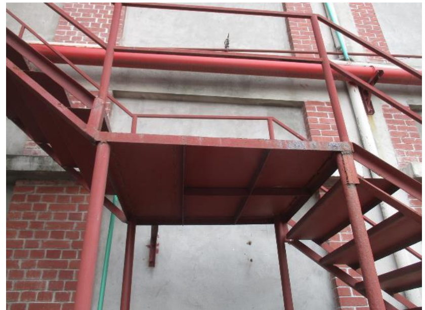
Poor connection of the external steel stair
