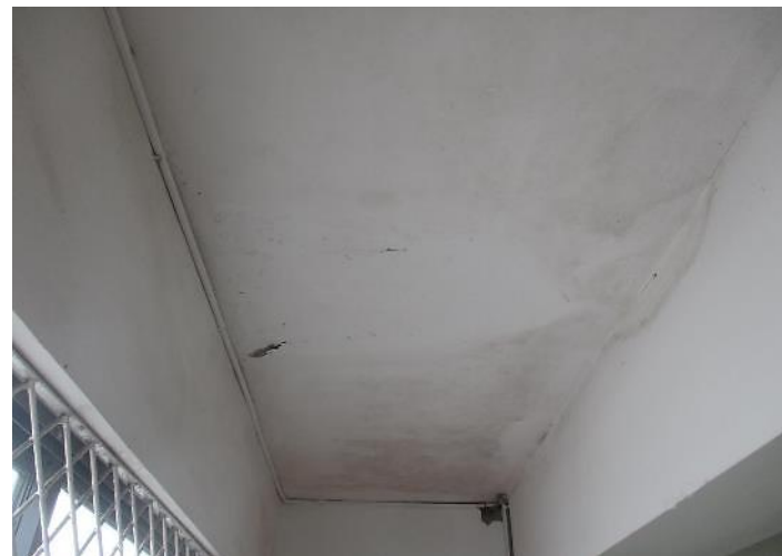
Dampness on soffit of stair roof slab
