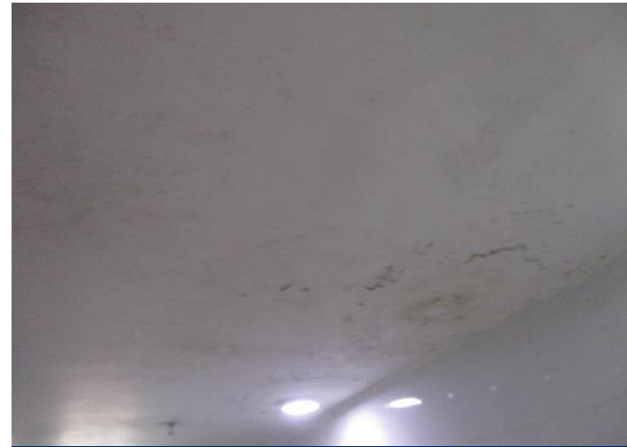
Dampness on soffit of toilet false slab
