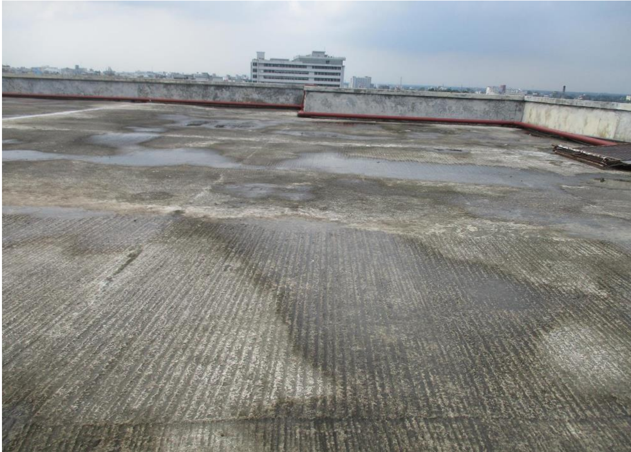
Stagnant water on the roof
