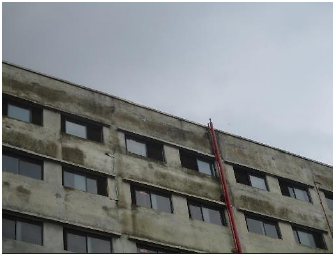
Dampness on exterior façade
