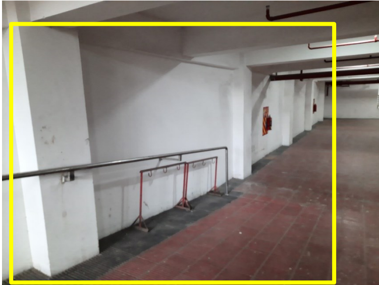
Columns at ramp area (semi-basement) are susceptible to impact loading from vehicles.
