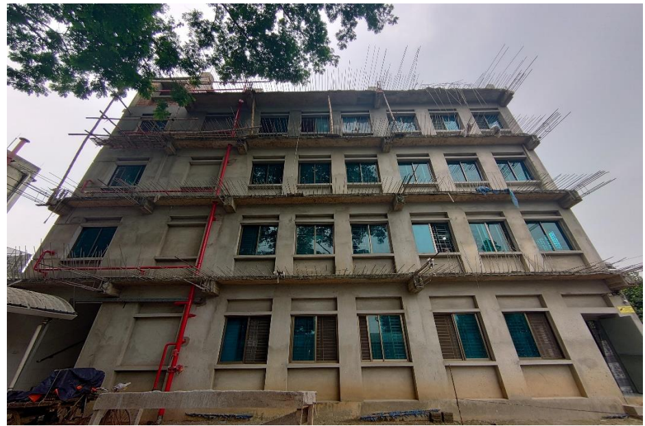
Exposed rebar of beam and slabs (south direction)
