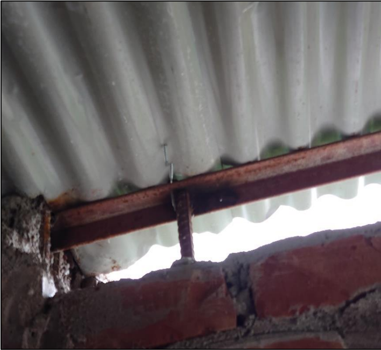
Poor connection details
