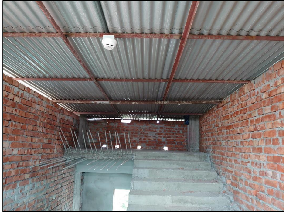
Apparently inadequate structural members
