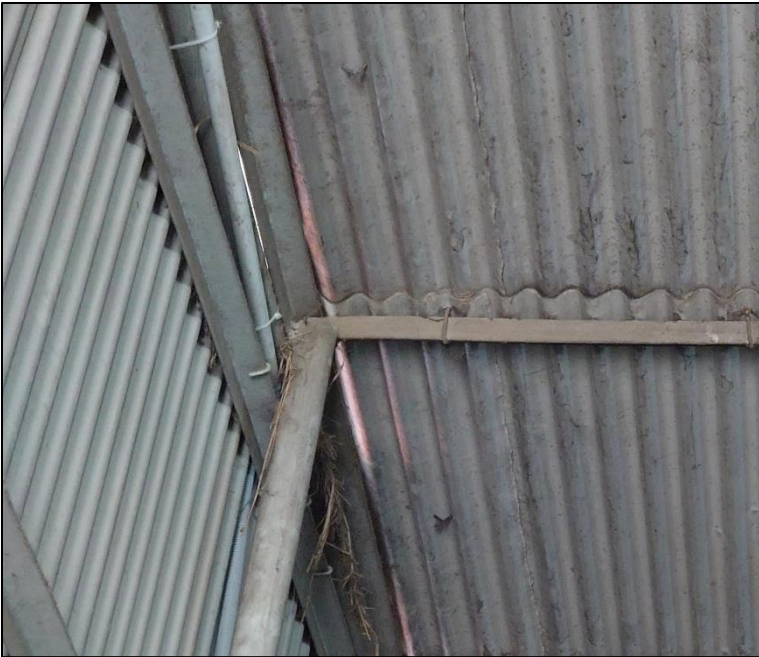
Poor connection details
