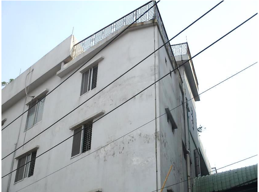
Dampness on exterior façade
