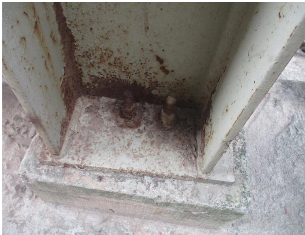
Corrosion on steel members
