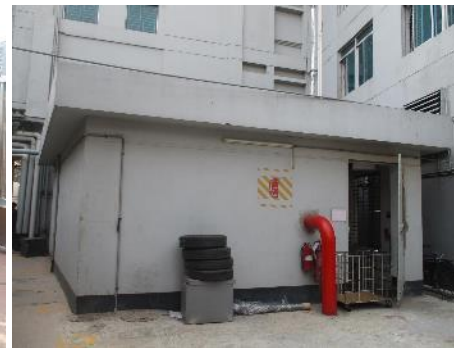
12. Fire Pump Room
