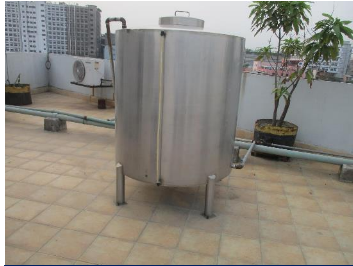
Roof- steel water tank (2000 L)
