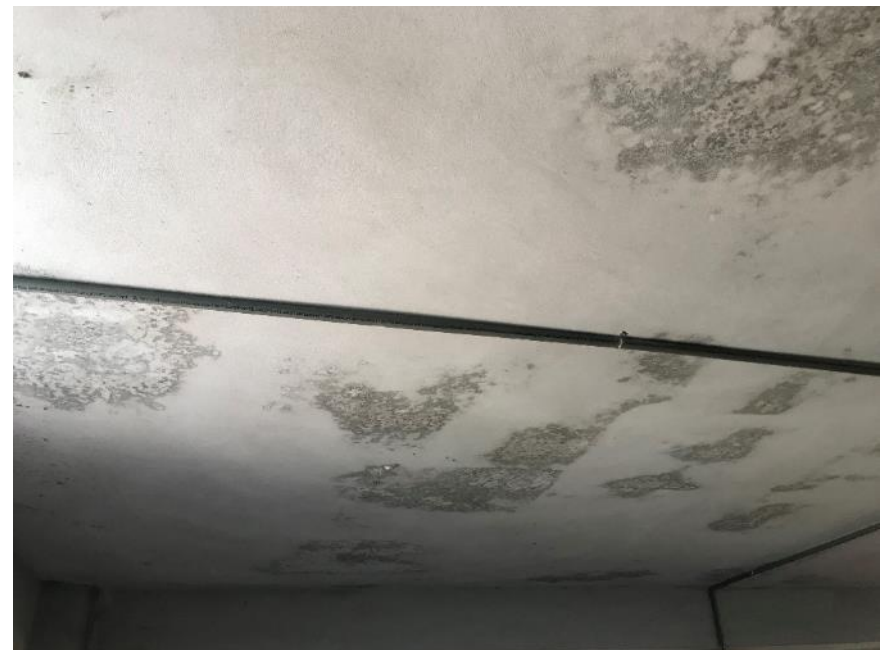
Dampness at Slab Soffit
