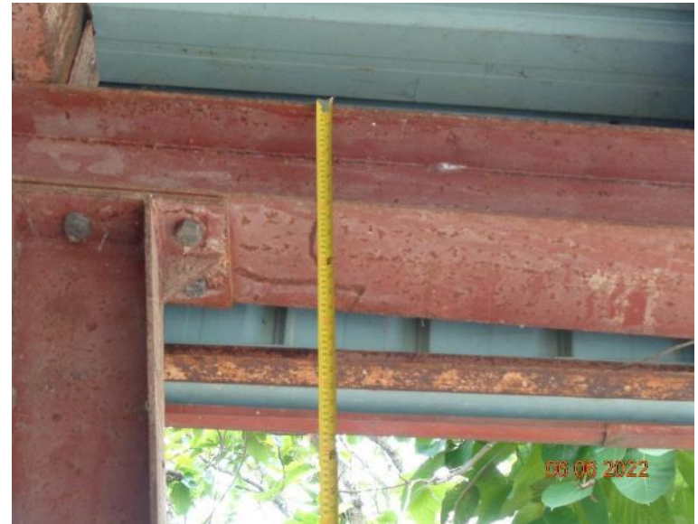
Corrosion in steel safter at Canopy
