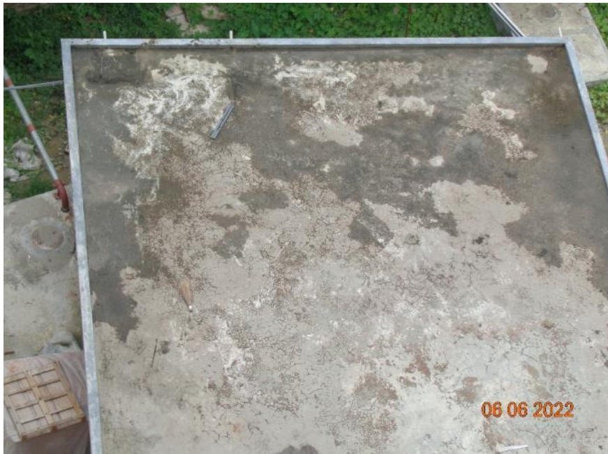
Water Ponding on Roof
