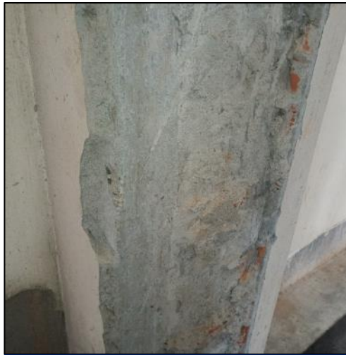
Stone Chips – Column Building-5
