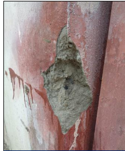
Stone Chips - Column (Building-7)
