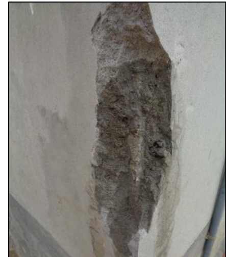
Stone Chips- Column (Building-6)
