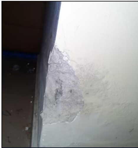
Stone Chips – Column Building-1
