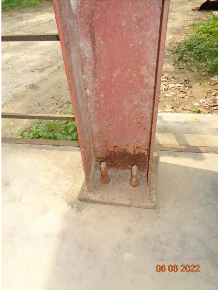
Corrosion in steel column (Canopy)
