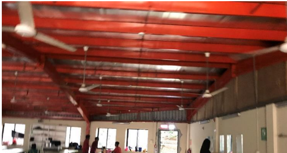
Compression strut missing
