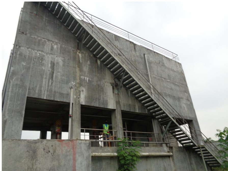
Apparently inadequate member size
