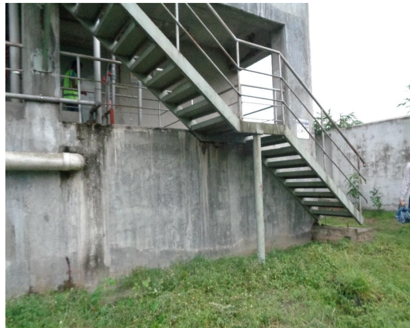
Apparently inadequate connection
