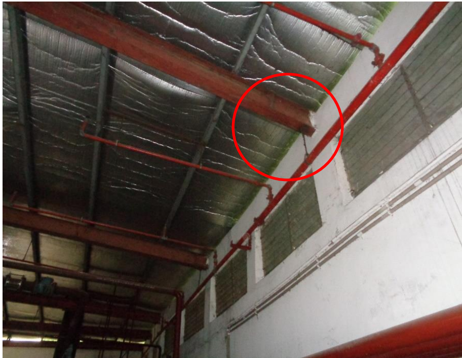
Apparently inadequate connection: rafter connected to brick wall (extended part)
