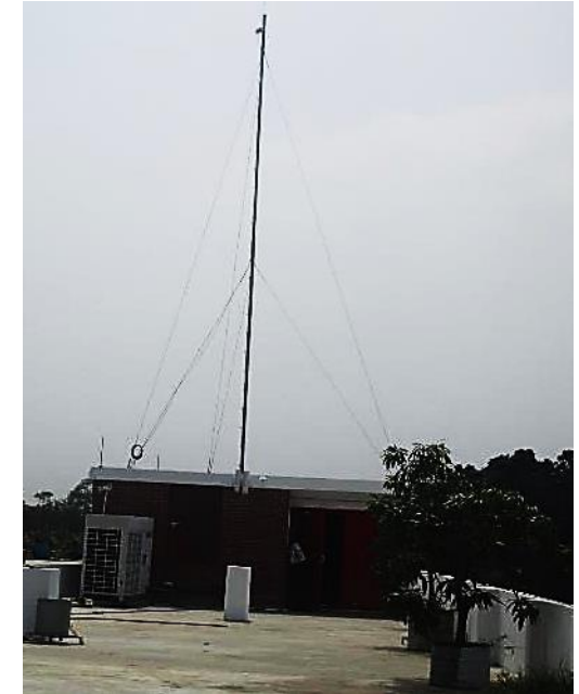
Telecommunication mast on the staircase.
