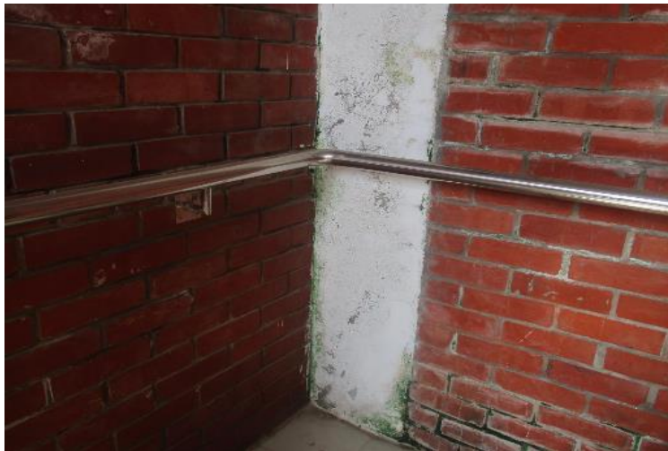
RC Column and wall in the staircase observed in damped condition due to the standing water.
