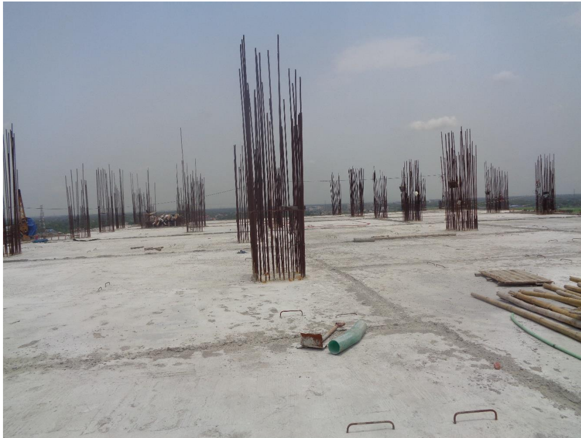
Exposed reinforcement left at roof
