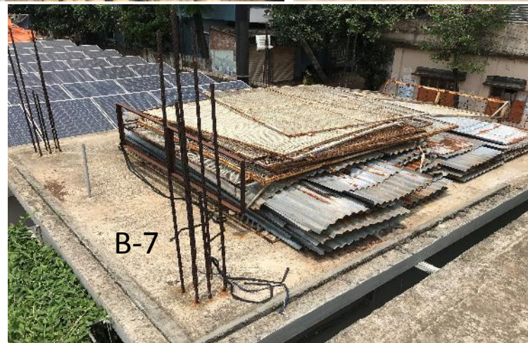
Falling hazard & construction debris on roof
