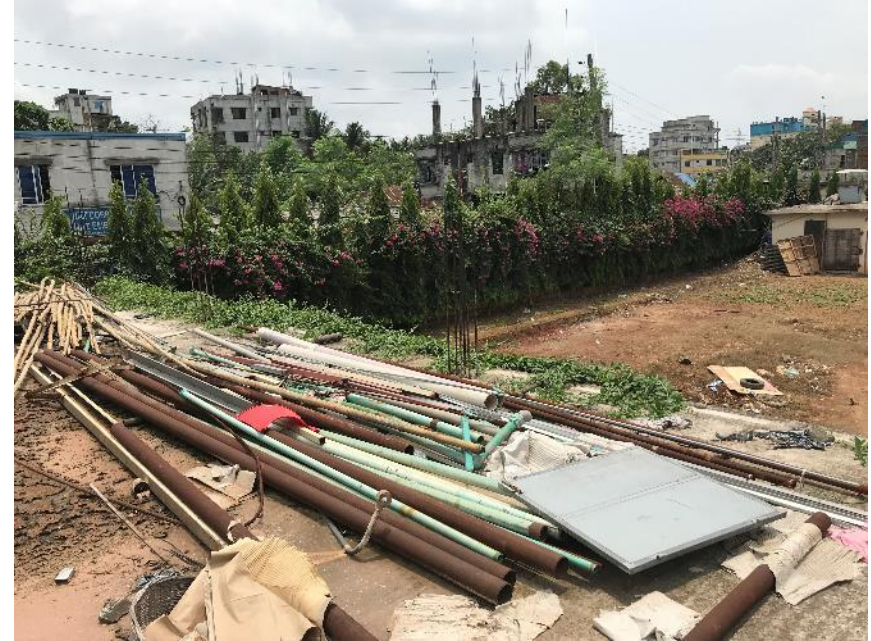
Blockage of drainage by construction debris
