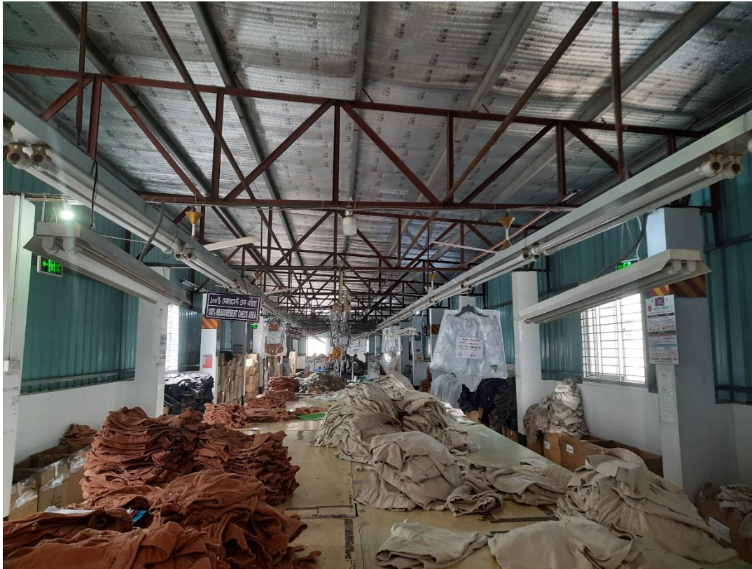
No roof bracing observed in the truss
