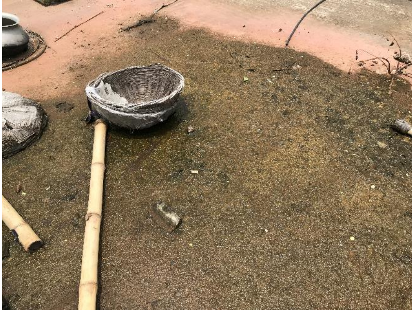
Water ponding on roof slab
