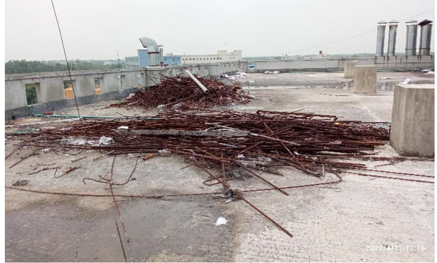
Construction debris on roof
