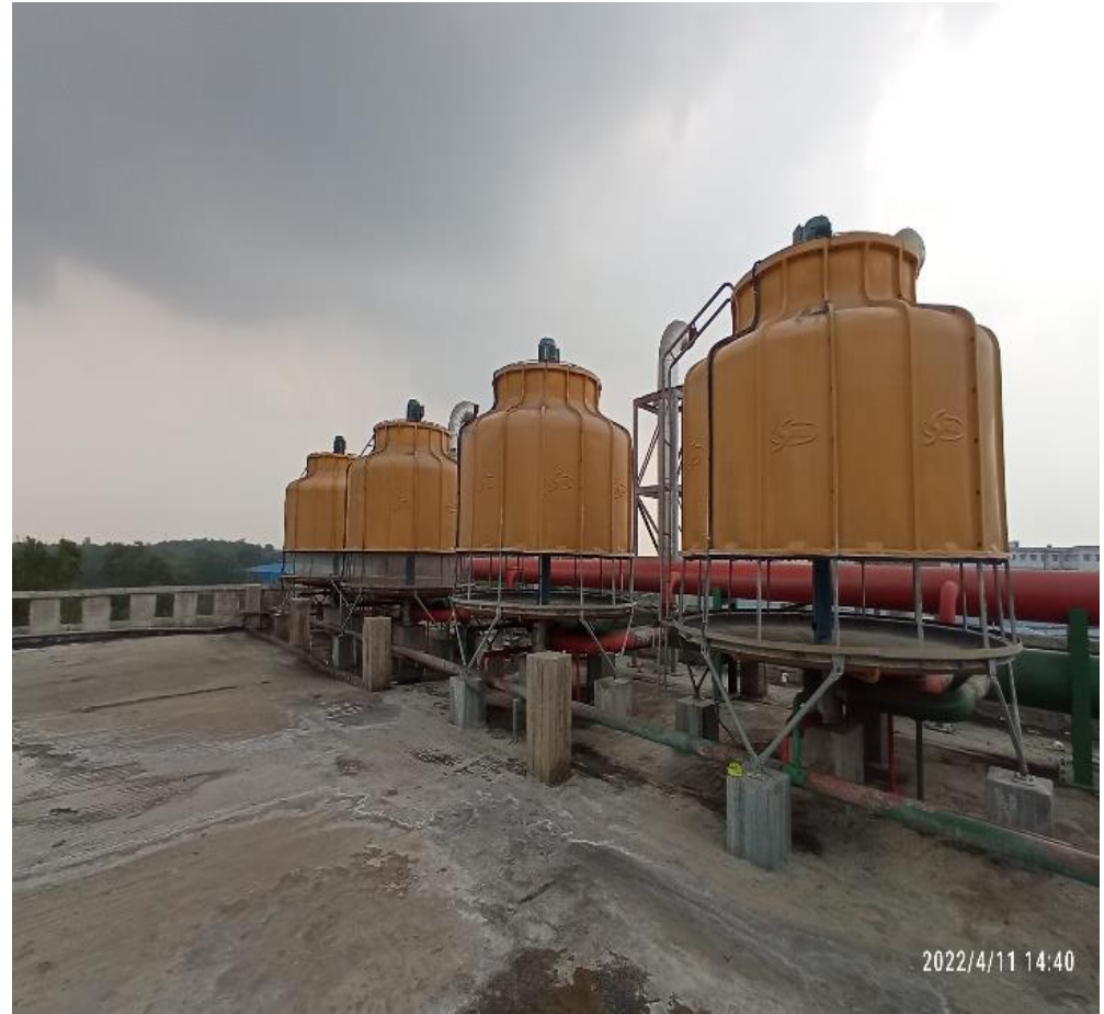
Chiller at roof
