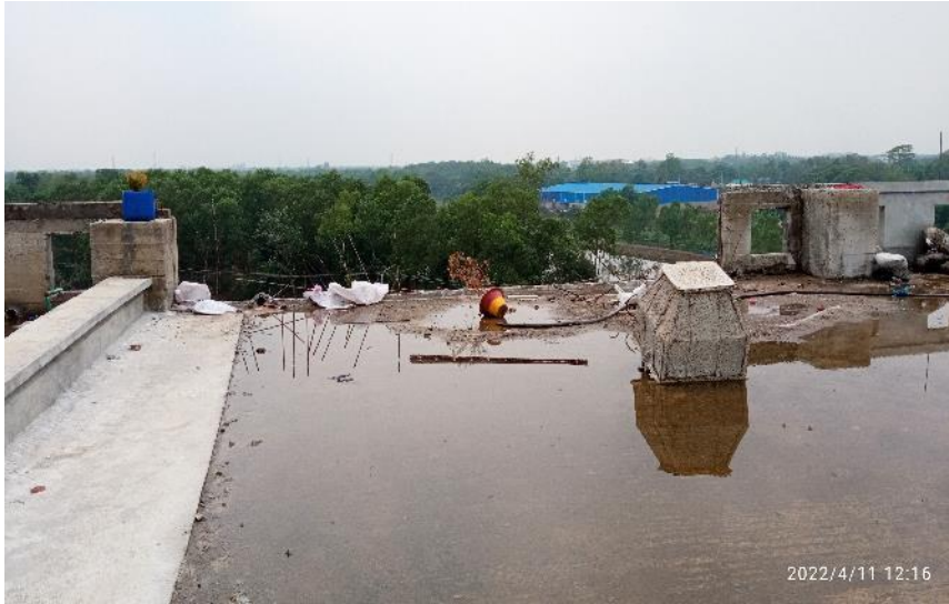
Falling hazard at roof
