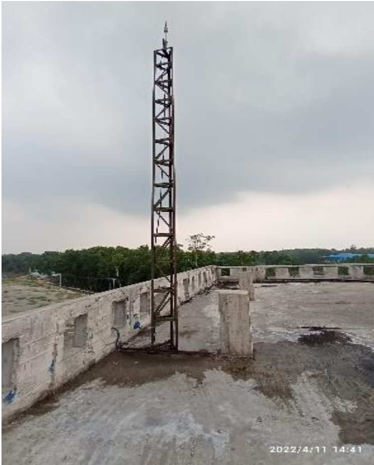
Telecom mast at roof
