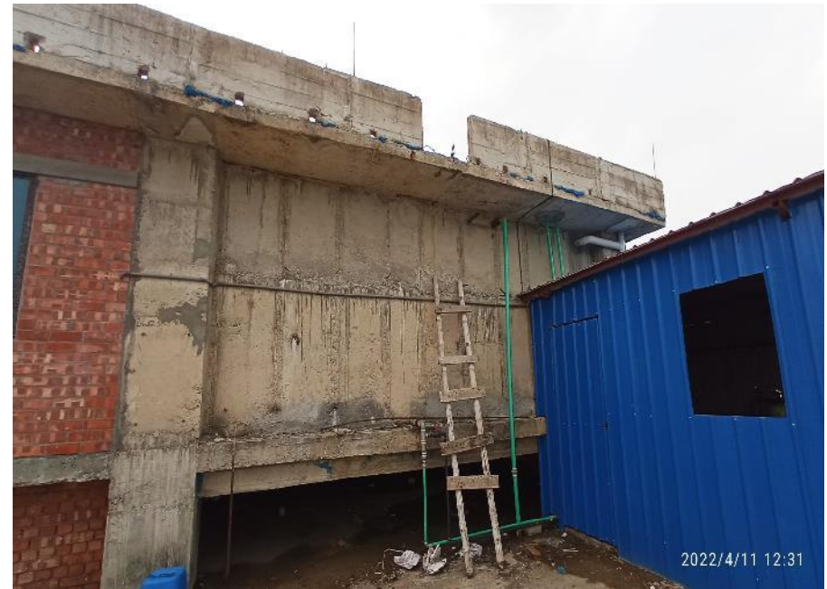
Water tank at roof
