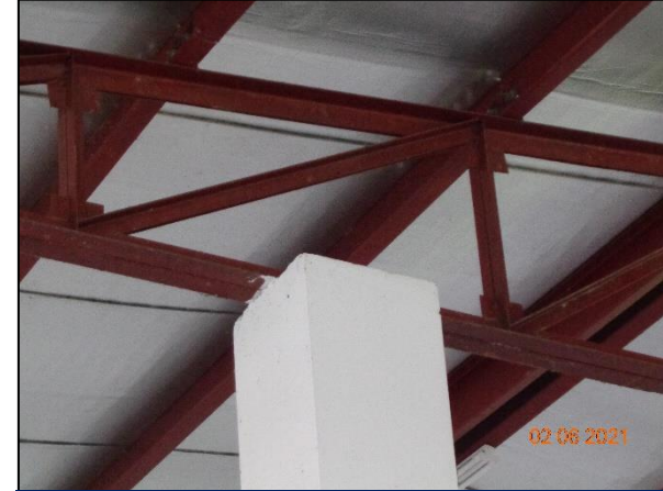
Poor connection details
