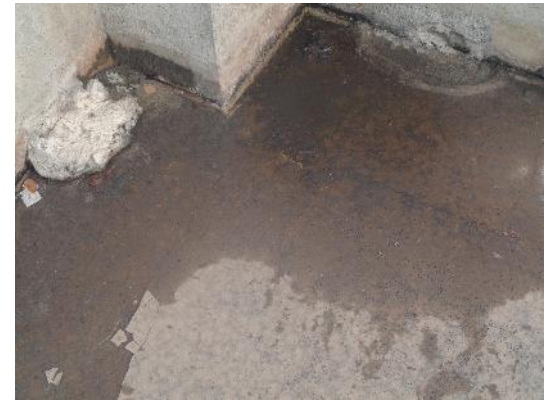
Water ponding at the roof of Building-2
