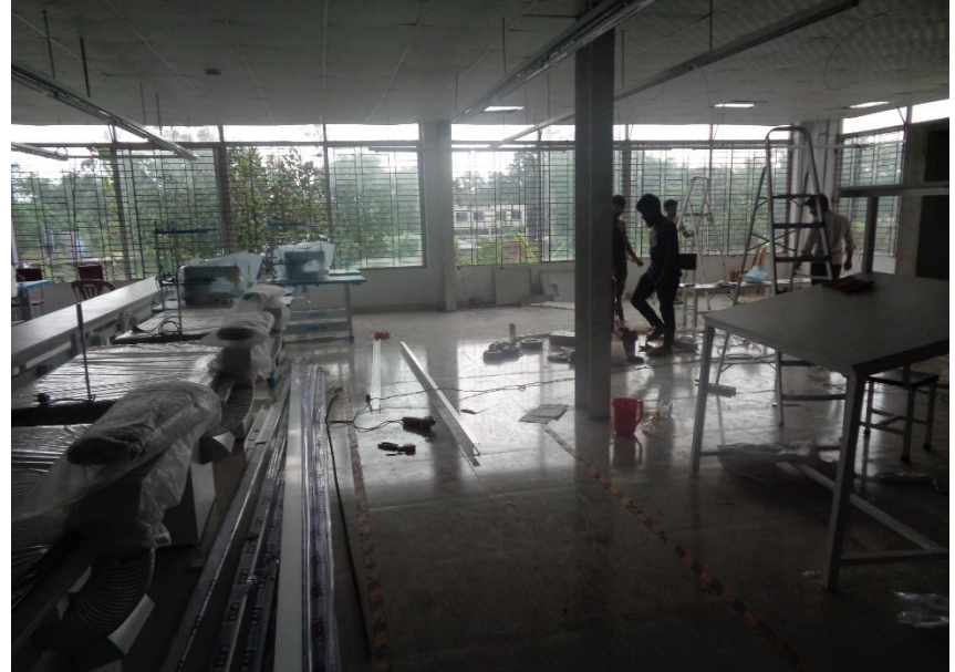
No wall bracing is provided
