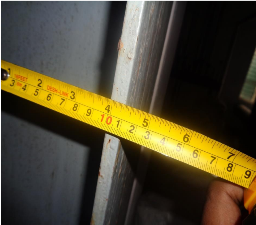
Flange thickness of column C-2 was measured as 10mm at ground floor
