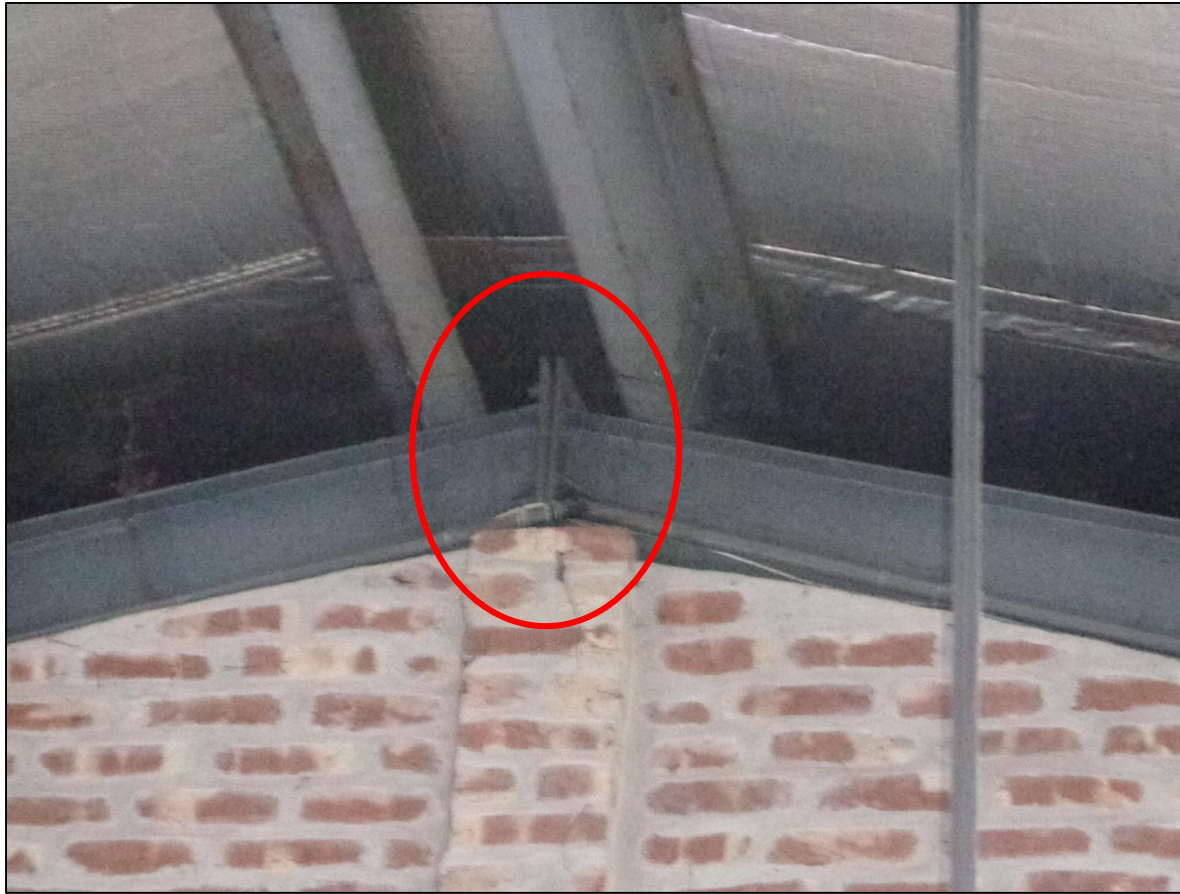
Significant gap in connection
