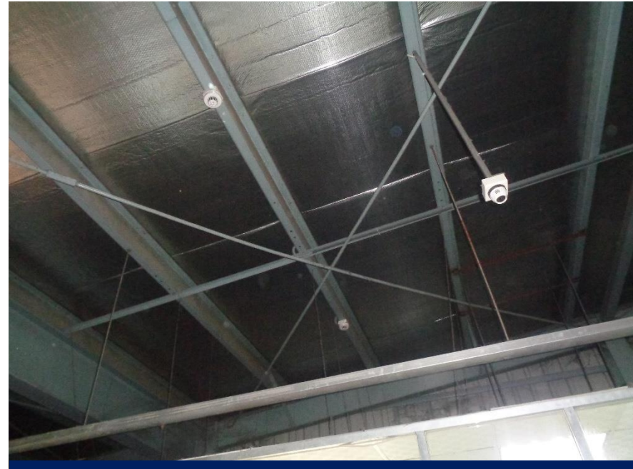
Loose rod bracing
