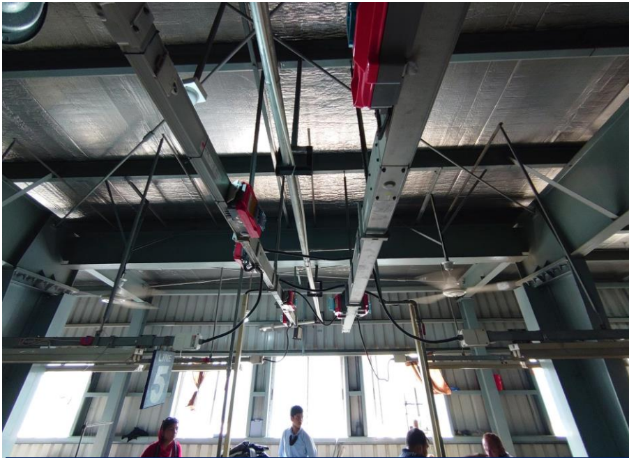
Loose rod bracing at roof
