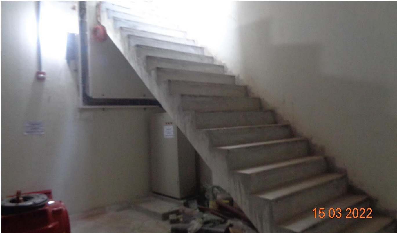
Falling hazard at pump room stair
