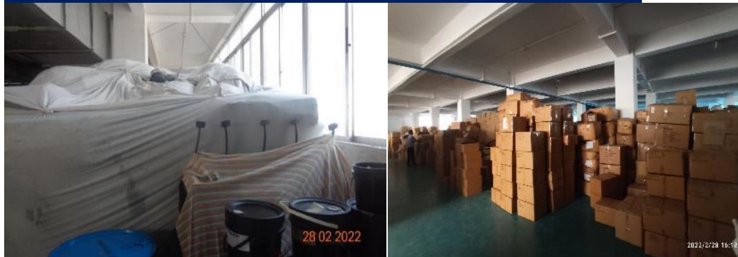
Uncontrolled loading on floors
