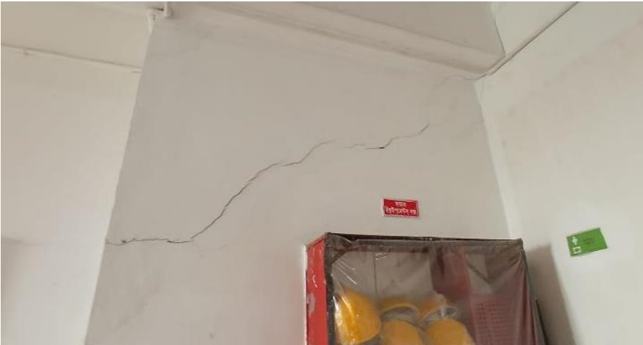
Fig- Crack on the brick wall
