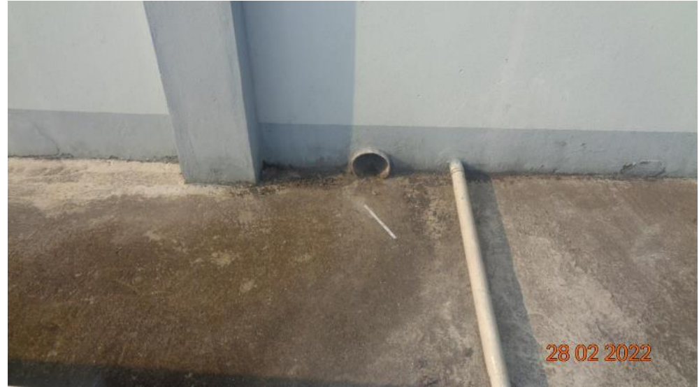
Signage of water ponding due to lack of proper sloping
