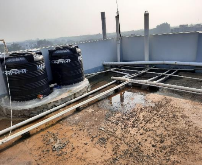
Water ponding on the roof slab
