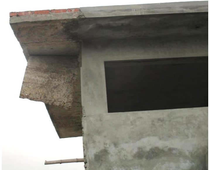
Hanging steel shutter
