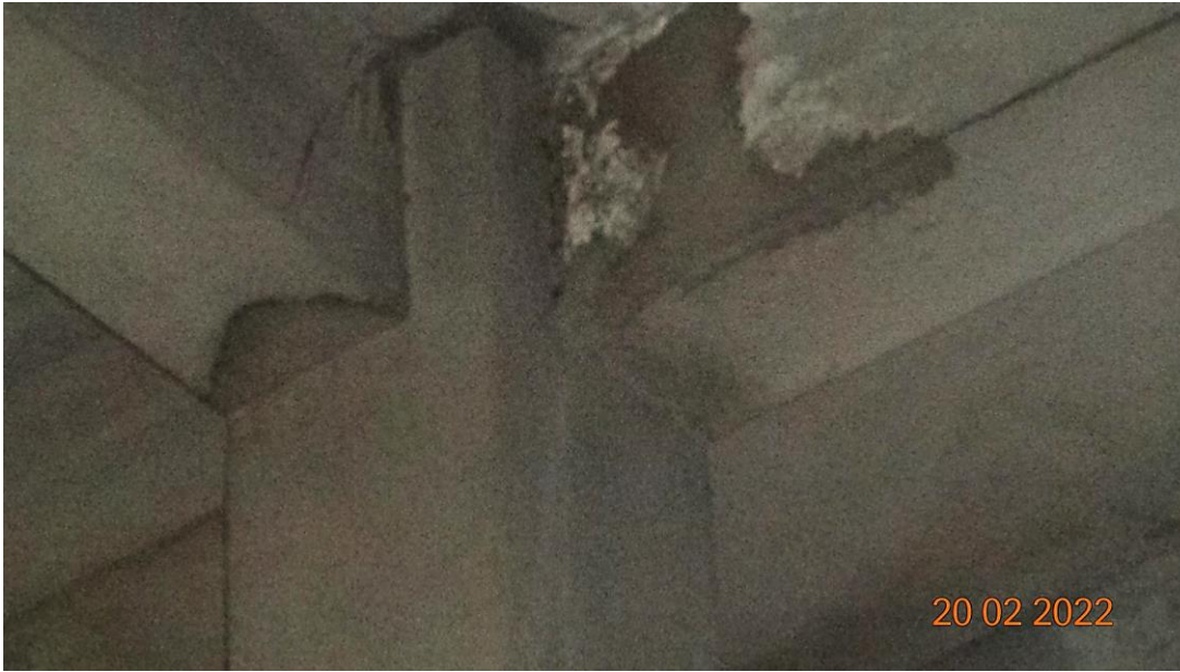
Water intrusion into the slab
