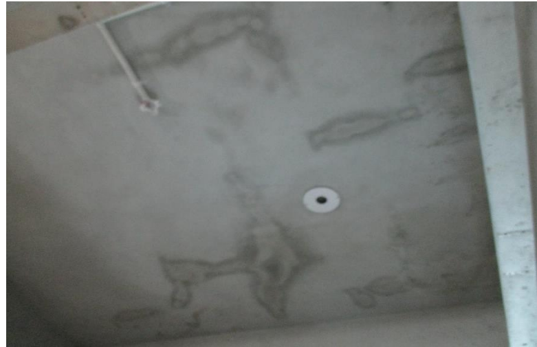
Sign of water intrusion into the roof slab
