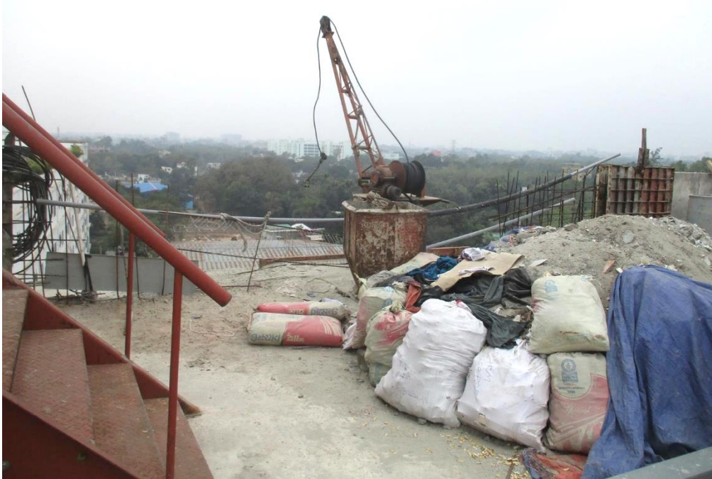
Incomplete parapet wall and construction debris
