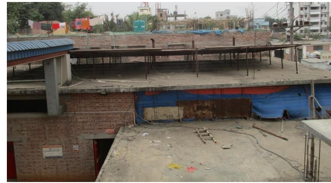
No water proofing layer on the roof
