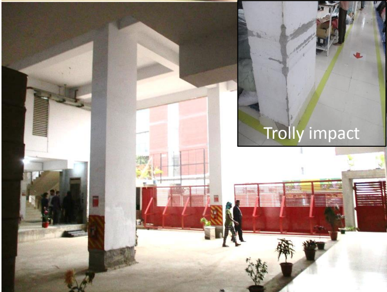
Ground floor column at loading-unloading zone is susceptible to vehicle impact
