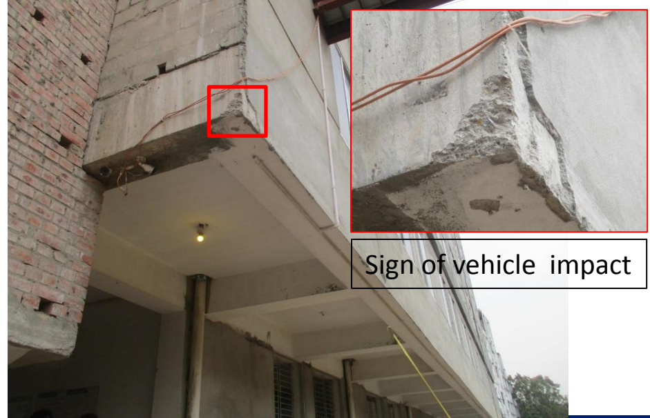
1st floor beam- susceptible to vehicle impact
