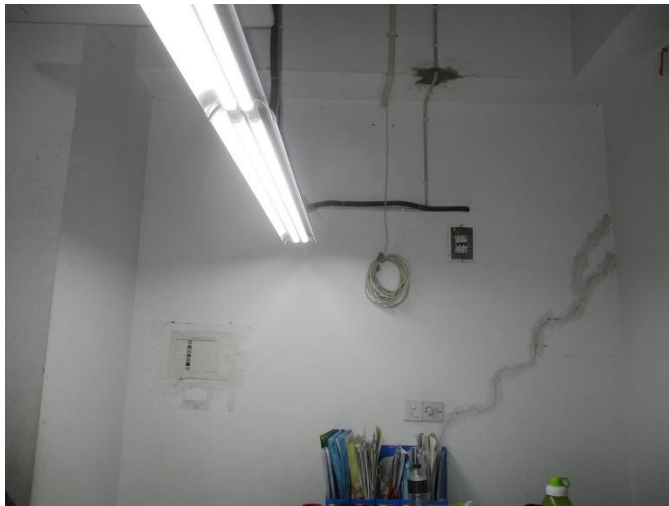
Crack in brick wall on cantilever area
