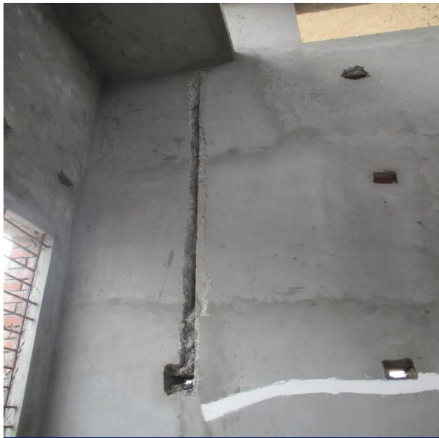
Crack in brick wall on stair landing
