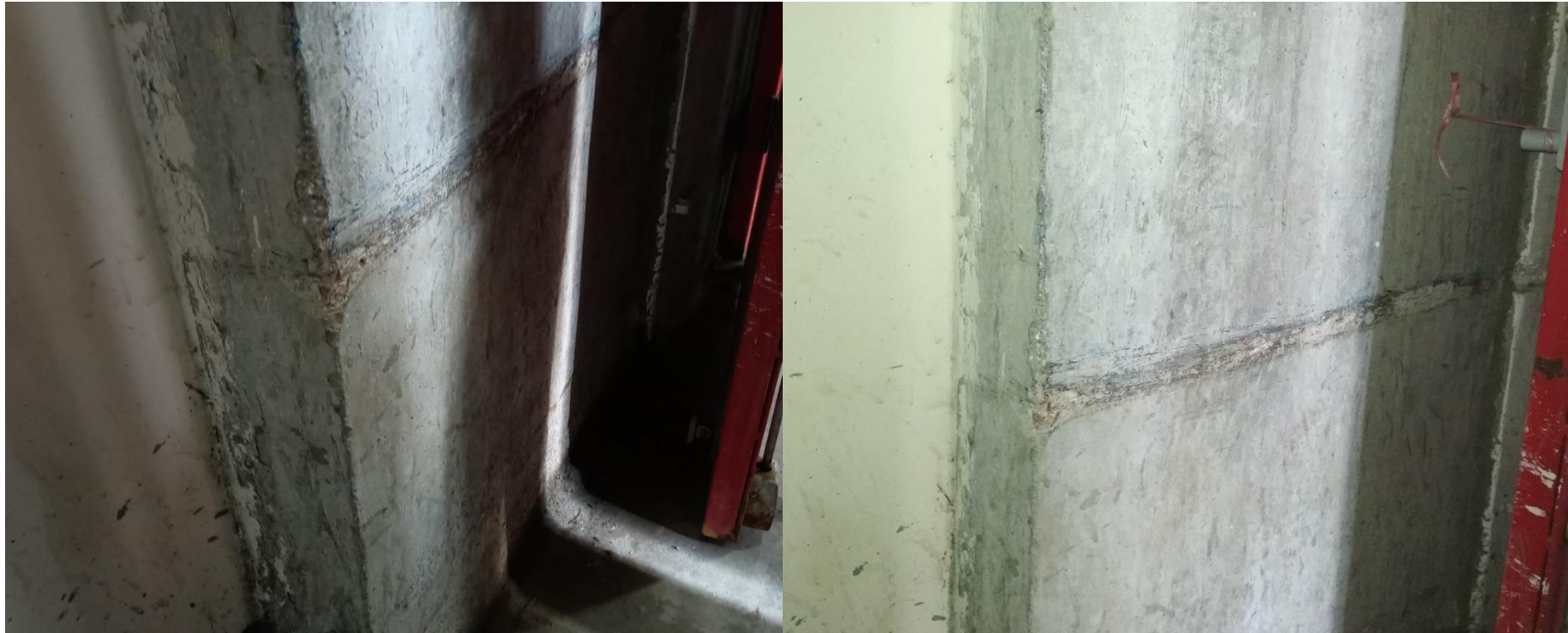
RC Column damaged due to impact of trolley
