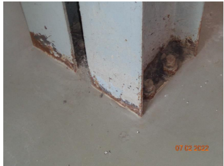
Corrosion in column
