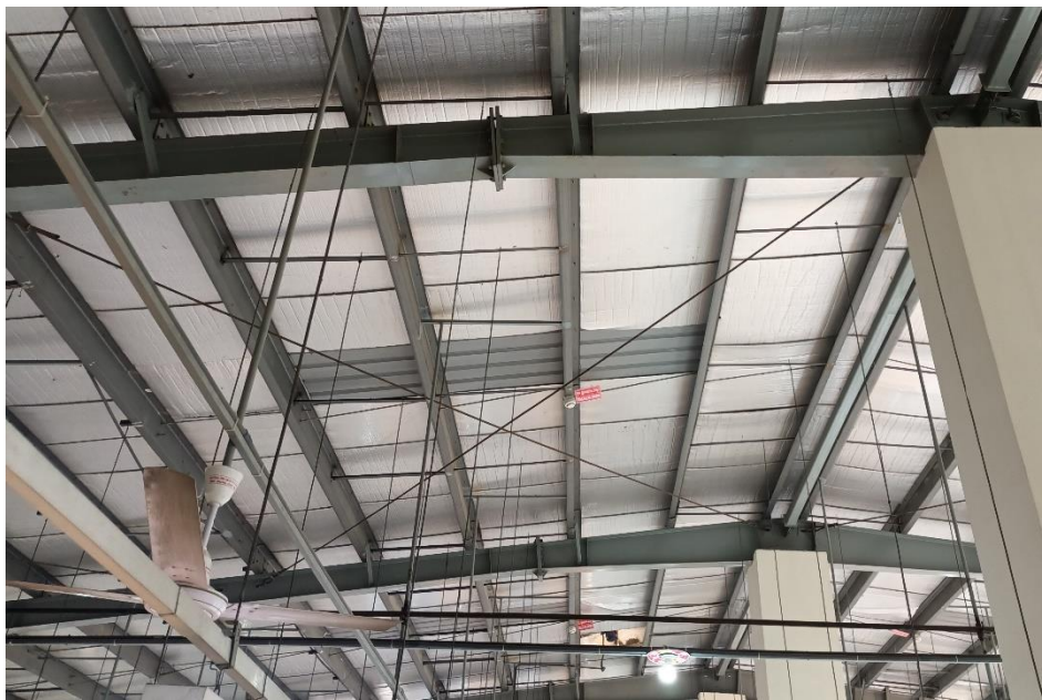
Loose cable bracing at roof
