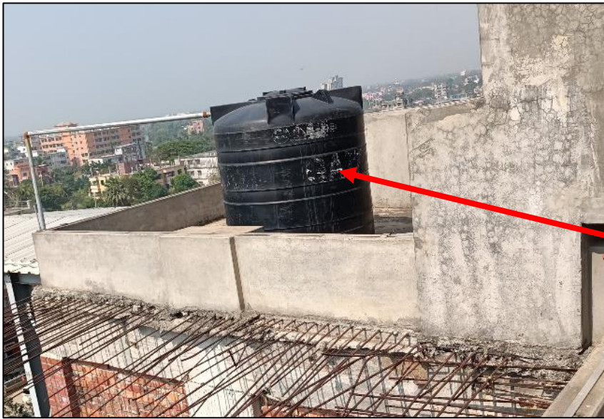
Undocumented 2000L water tank
