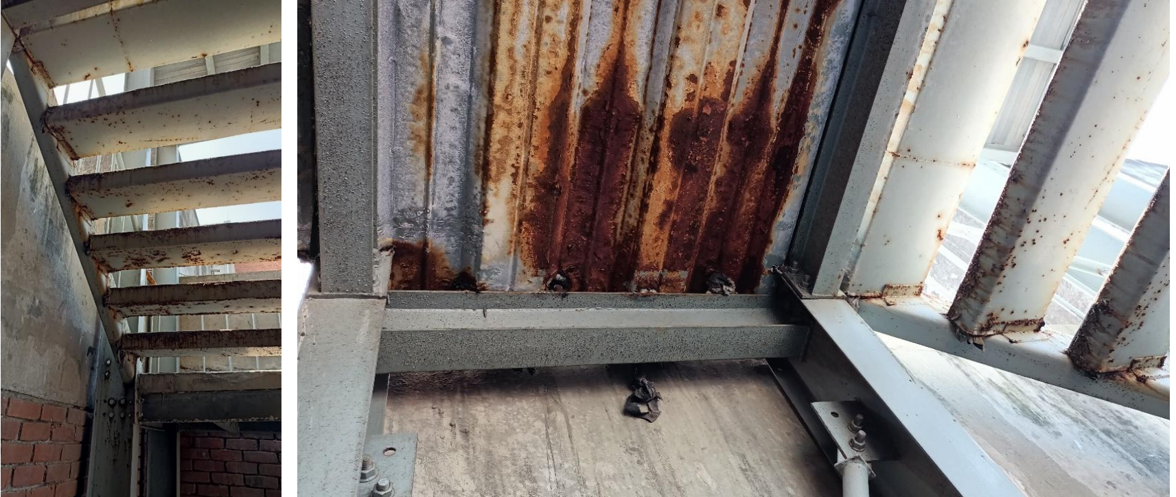
Corrosion in steel member of steel stair
