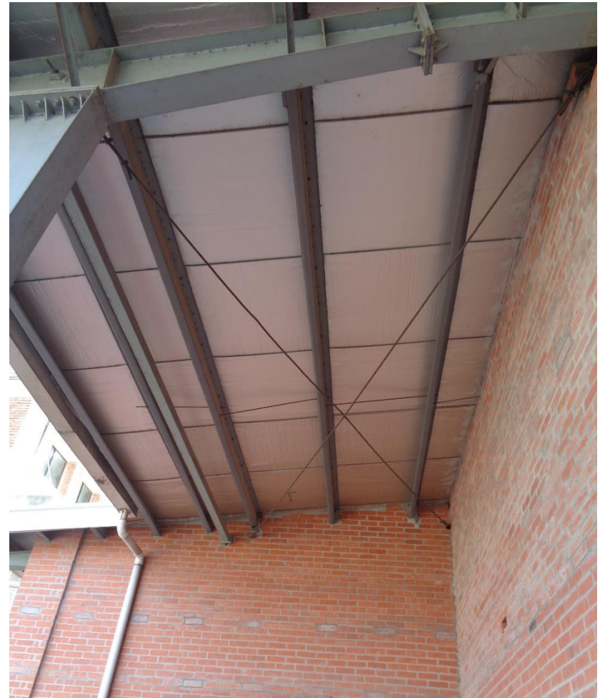
Loose cable bracing
