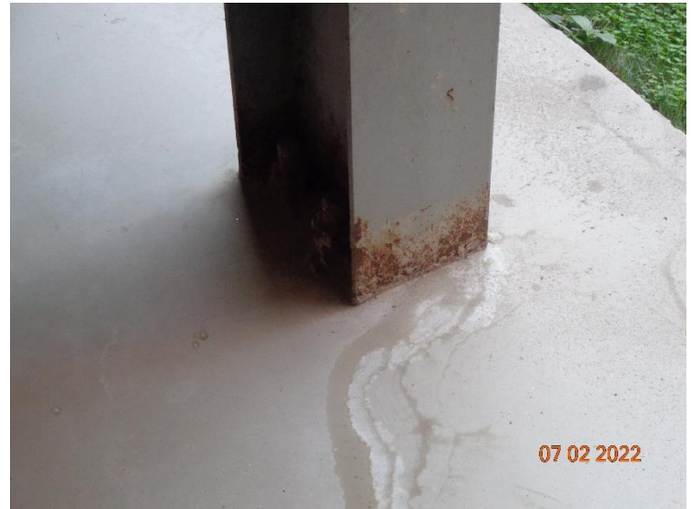
Corrosion in Column
