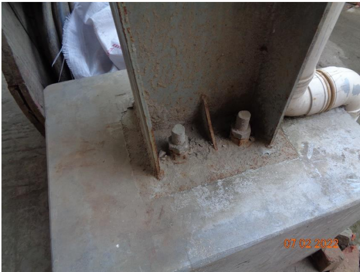
Corrosion in Base Plate
