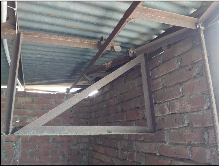
Poor connection details
