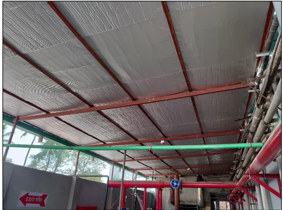
Apparently inadequate structural members
