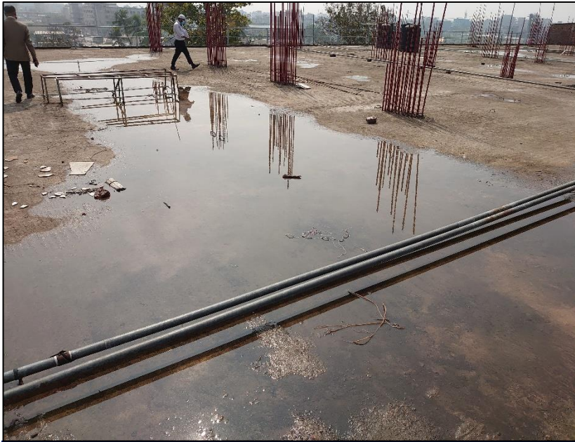
Water ponding on the roof
