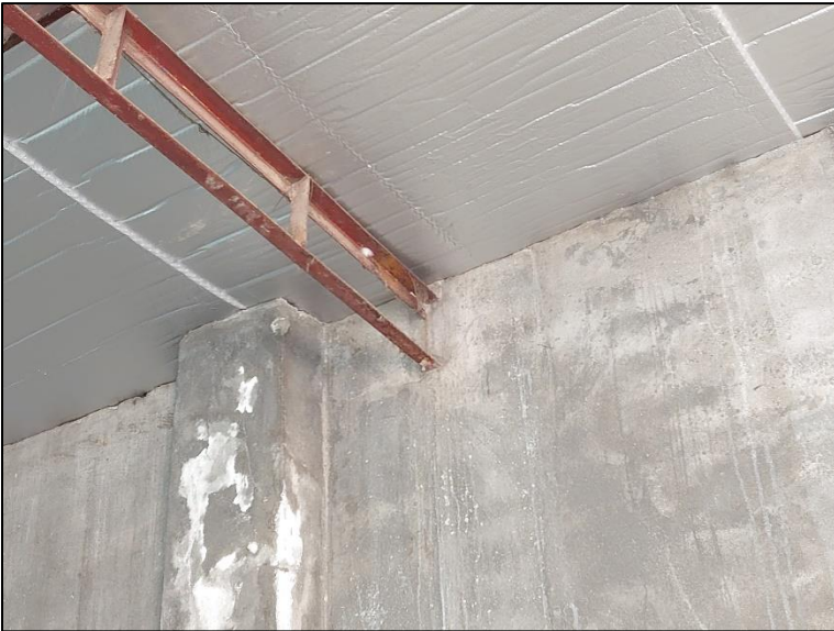
Poor connection details
