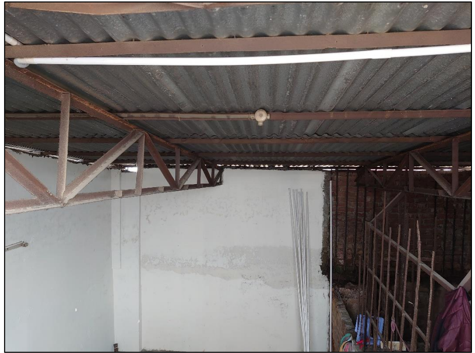
Inadequate structural members
