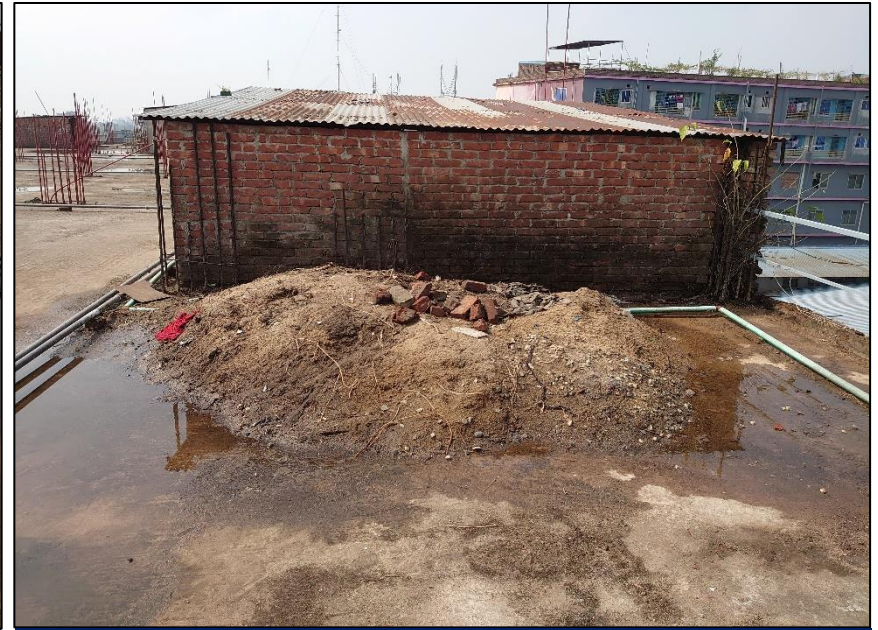
Construction debris on the roof
