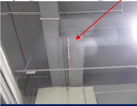
Water damage on beam
