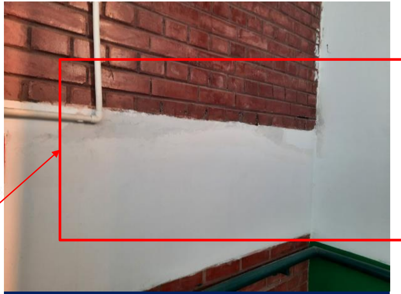
Water damage on beam & column
