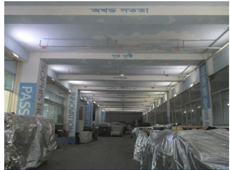
Ground floor column susceptible to vehicle impact
