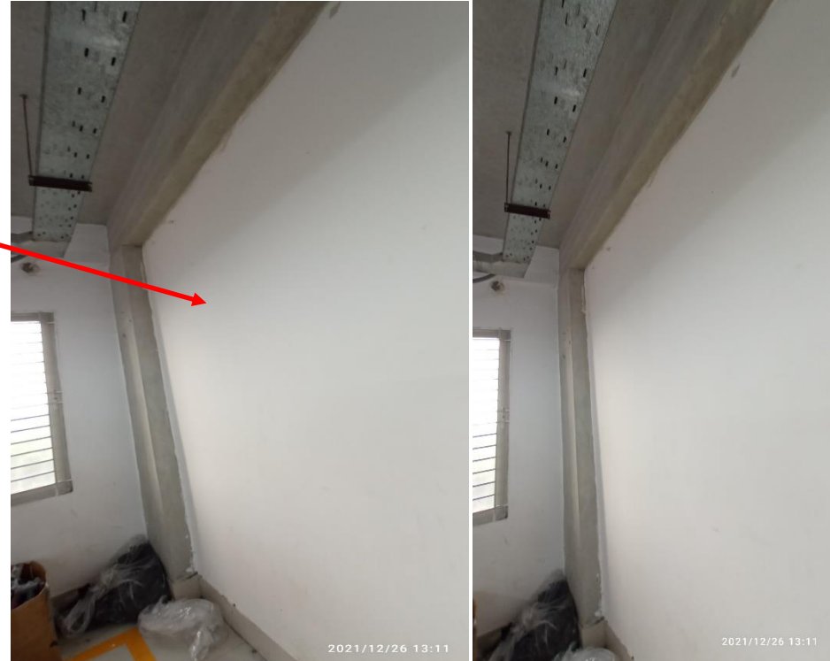
Missing shear wall at 5th floor. Brick wall constructed instead of RC shear wall
