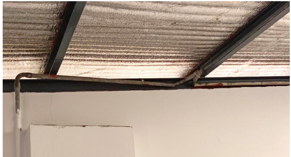
Non engineered connection
