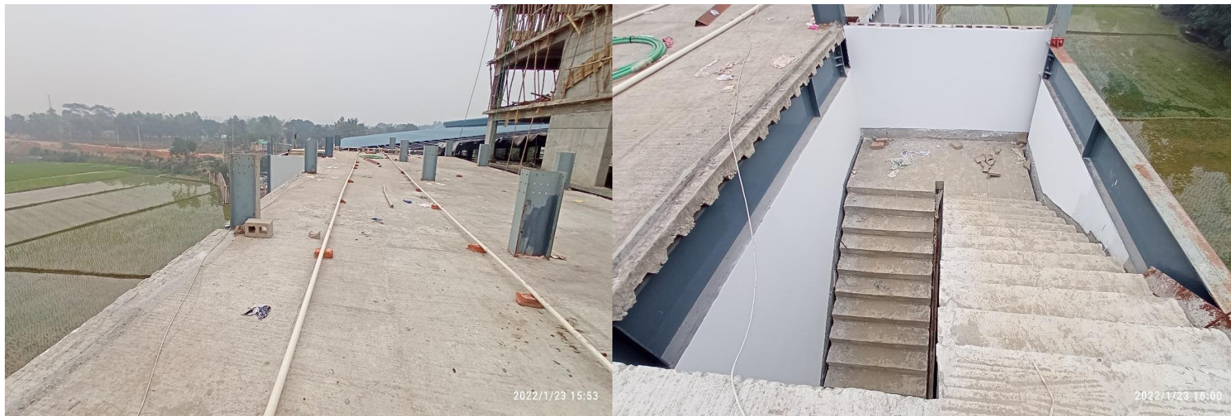
No parapet/barrier on roof & stair
