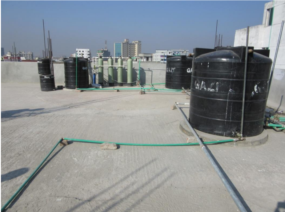
Water tanks on roof
