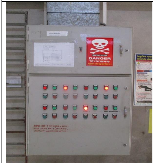
Typical electrical distribution panel.
