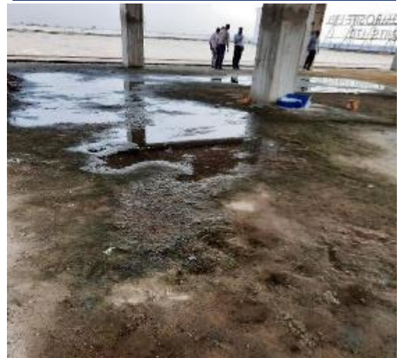
Incomplete finishing works at roof
