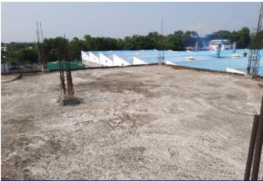
No parapet on roof
