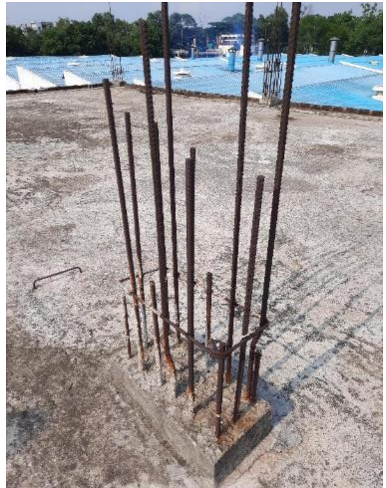
Exposed rebar prone to be corroded
