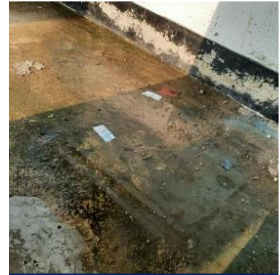
Stagnant water at roof
