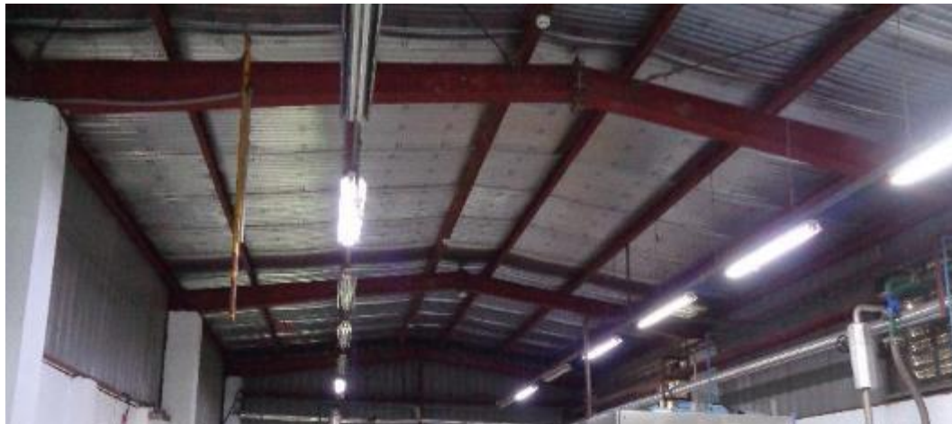
Roof bracing only in one bay
