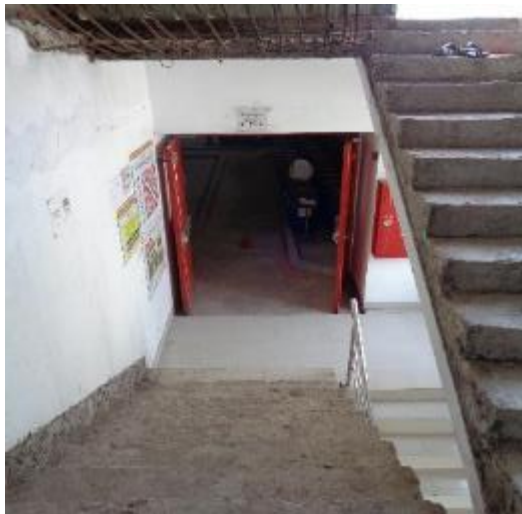
No guardrails around the stair
