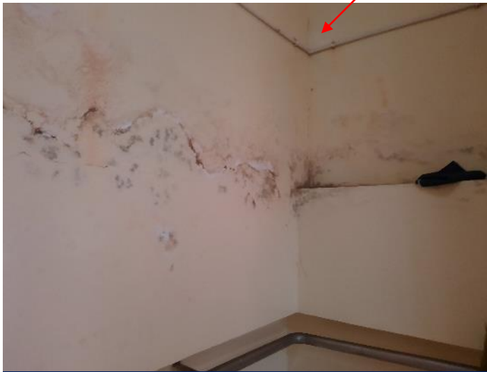
Dampness on 4 th floor staircase
