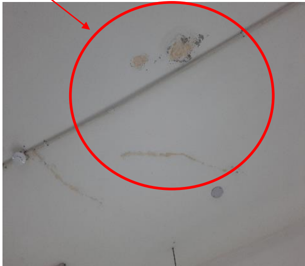
Dampness on 1 st floor roof
