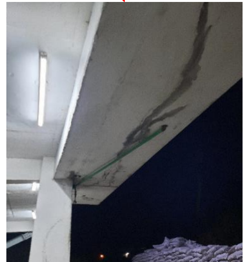
Dampness on ground floor
