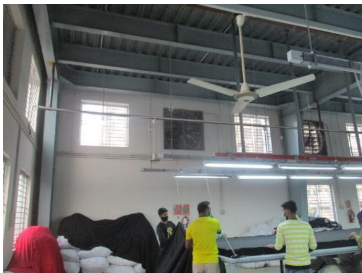
No vertical bracing at wall
