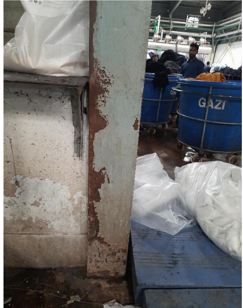
Corrosion in column
