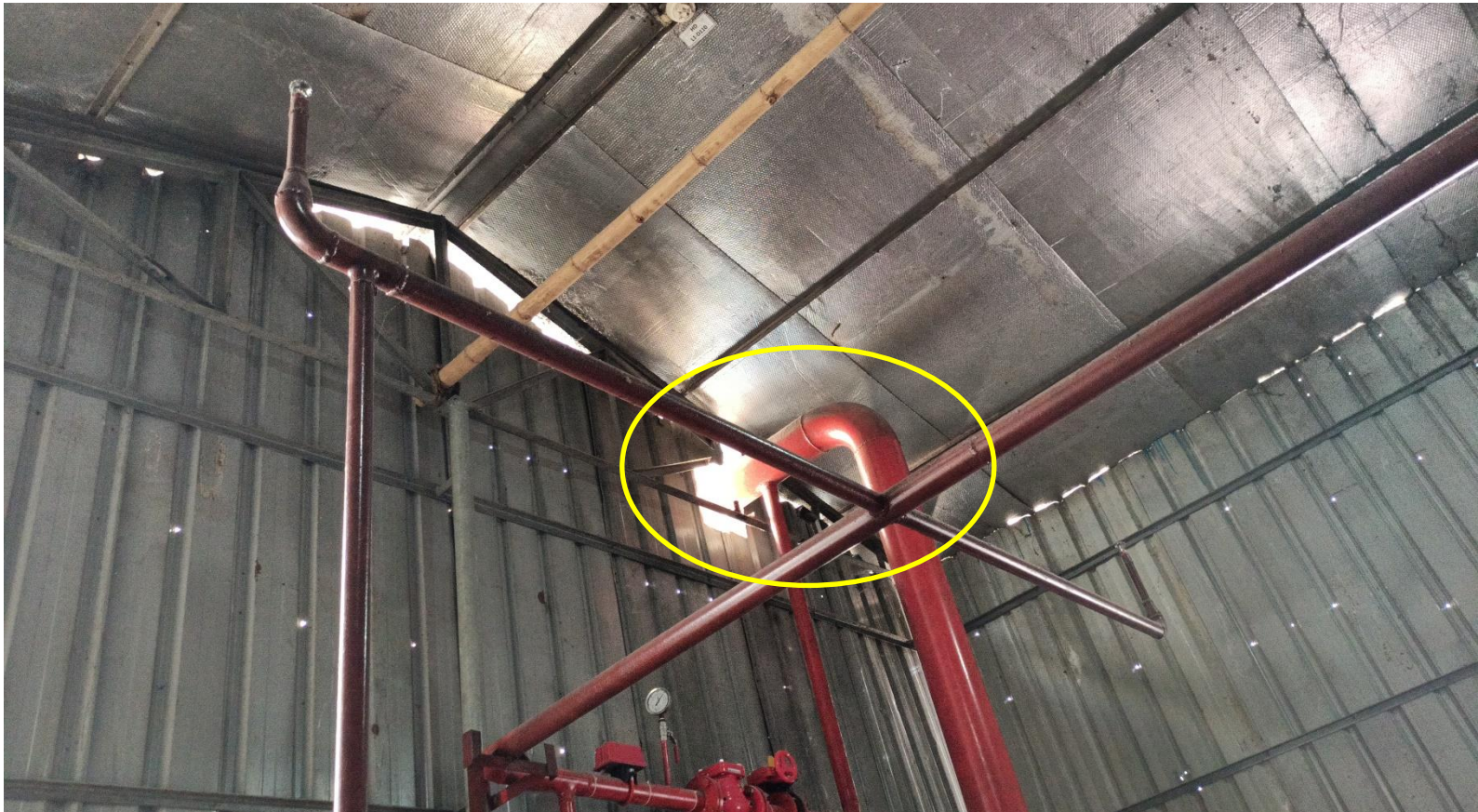
Discontinuous truss member
