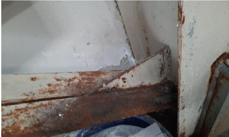
Corrosion in Bracing
