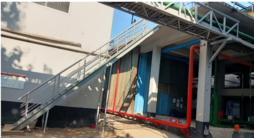
Apparently inadequate steel member size and no stability system provided.
