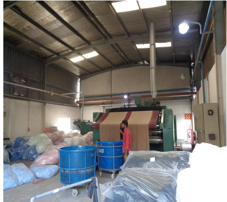
No load transfer media provided; wall/roof bracing not provided at rest of the bays
