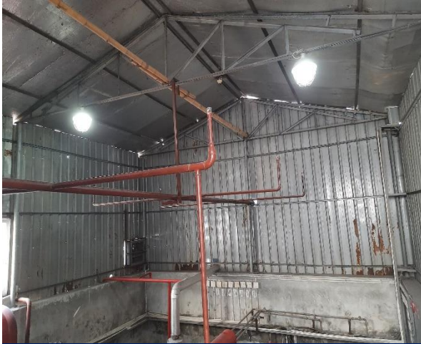
B-17: Fire Pump Shed
