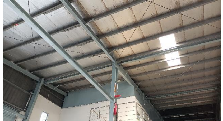
Loose cable bracing
