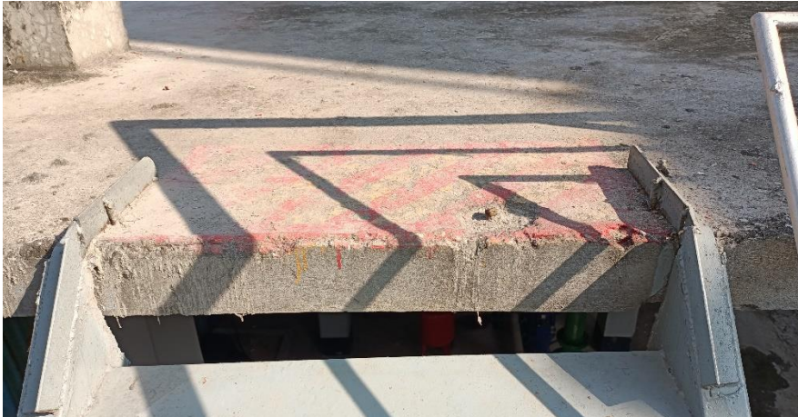
Apparently inadequate connection
