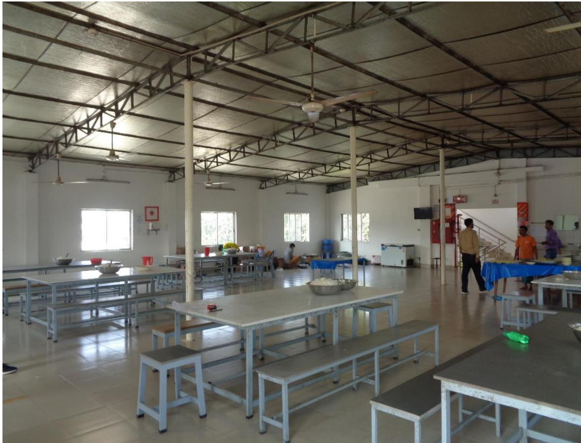
No bracing system/load transfer media provided
