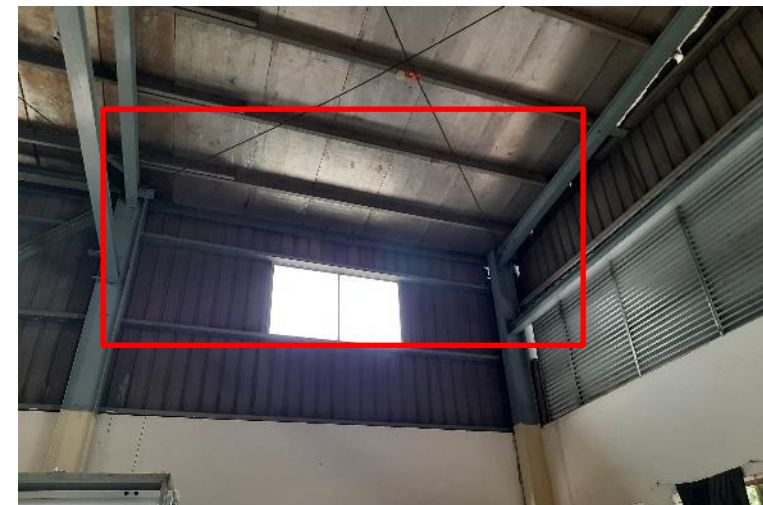
No compression member at grid 17~18
