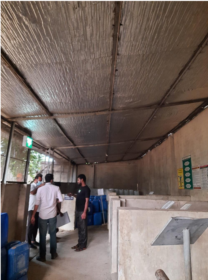
No clear load path with poor connection
