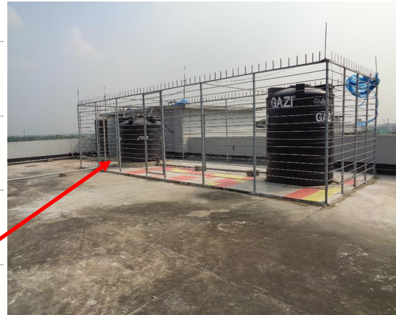
Plastic water tank (5000 liter each)
