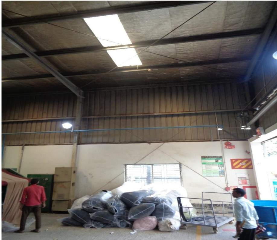
Wall/roof bracing provided at only one bay
