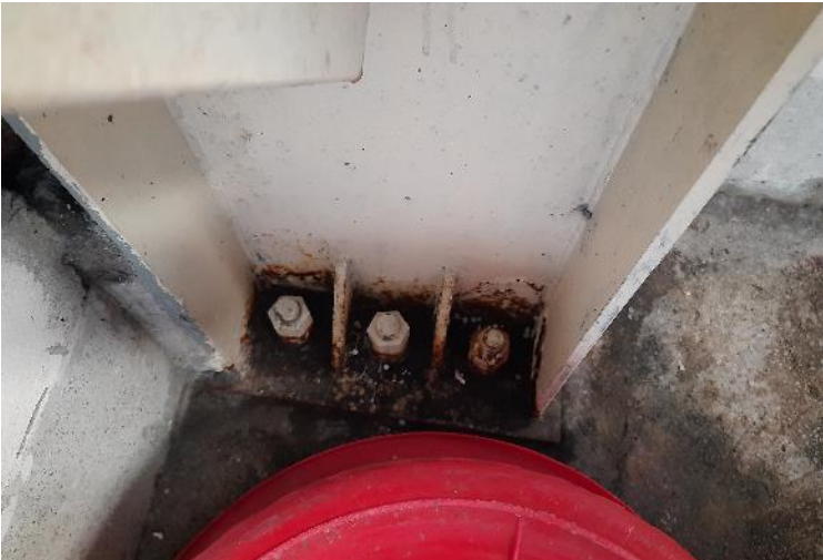
Corrosion in Base Plate
