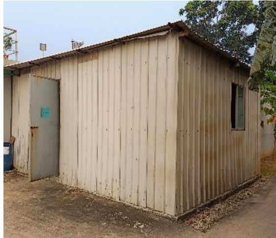
B-18: ETP Sludge M/C Room
